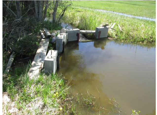
Figure 4.4-26. Example Pre-Cast Concrete Splitter Structure.
