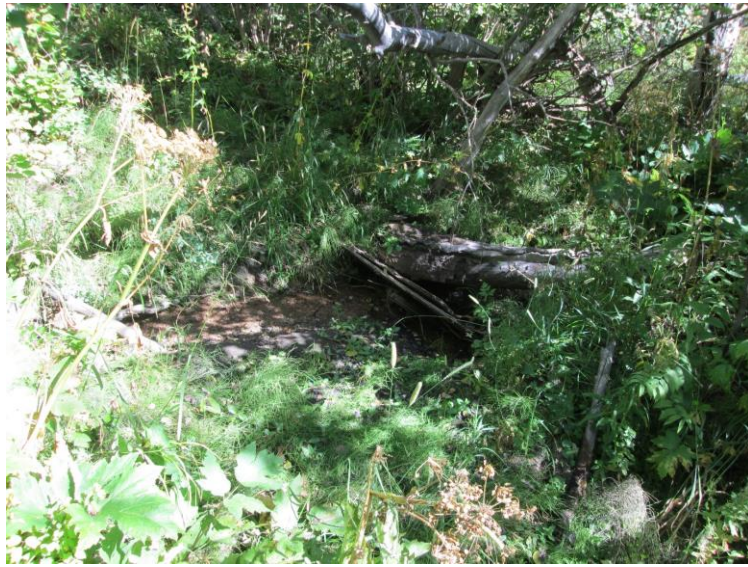
Figure 4.4-14 Simon Johnson 2 Ditch Diversion Structure.
