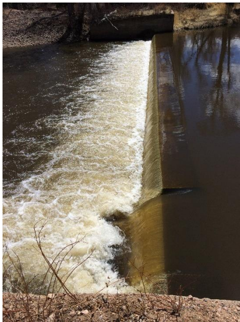
Figure 3.6-12 Pioneer Canal Diversion Structure.
