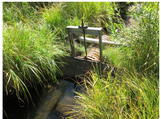
Figure 4.4-12 Simon Johnson Ditch Diversion Structure.
