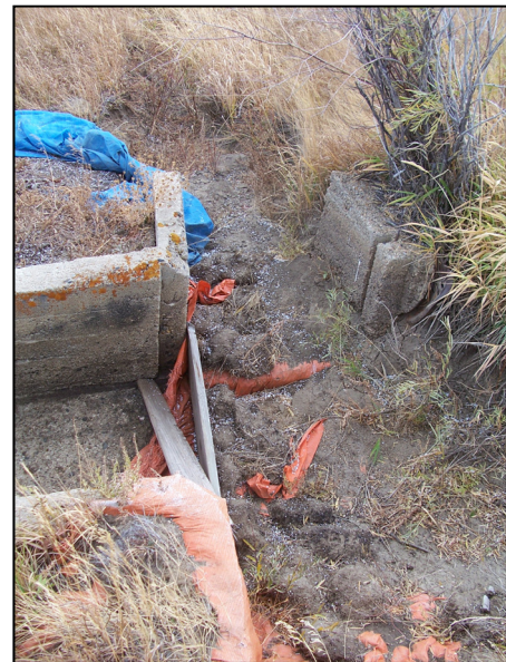
Figure 2.36 Splitter Box in Poor Condition on Graham and Farnsley Ditch No. 1.
