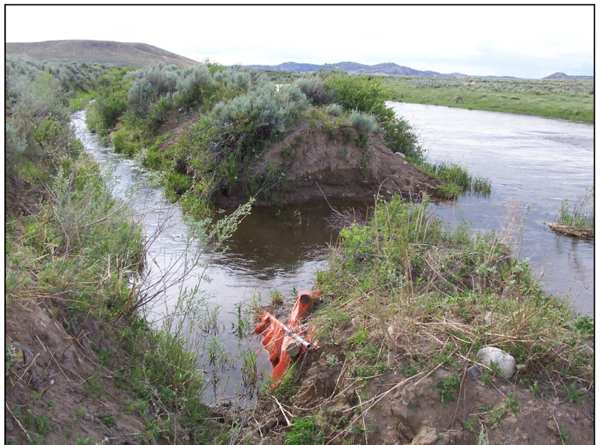
Figure 2.36 Cranor Ditch Failure on the Sweetwater River.
