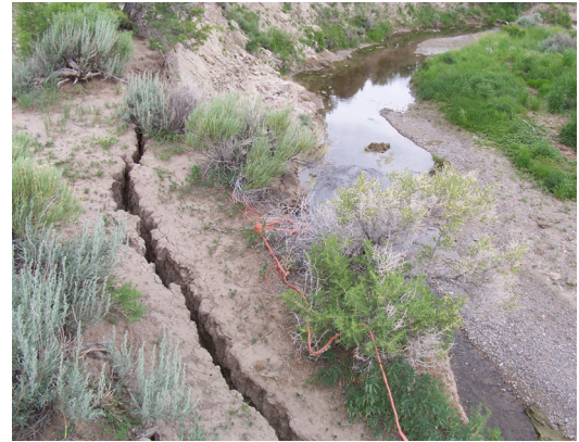
Figure 2.23 Stream Bank Instability on Lower Dry Creek.
