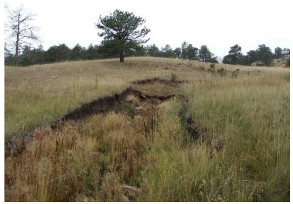
Erosion in Emergency Spillway
