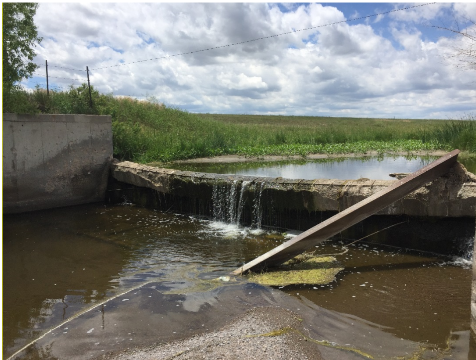
Beaver Dam Ditch Diversion, Example of Partial Fish Passage Barrier on Crow Creek
