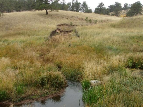
Erosion in Emergency Spillway
