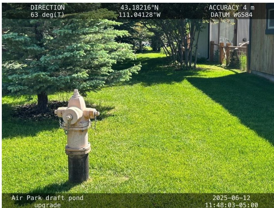
Figure D-31. Existing drafting station.
