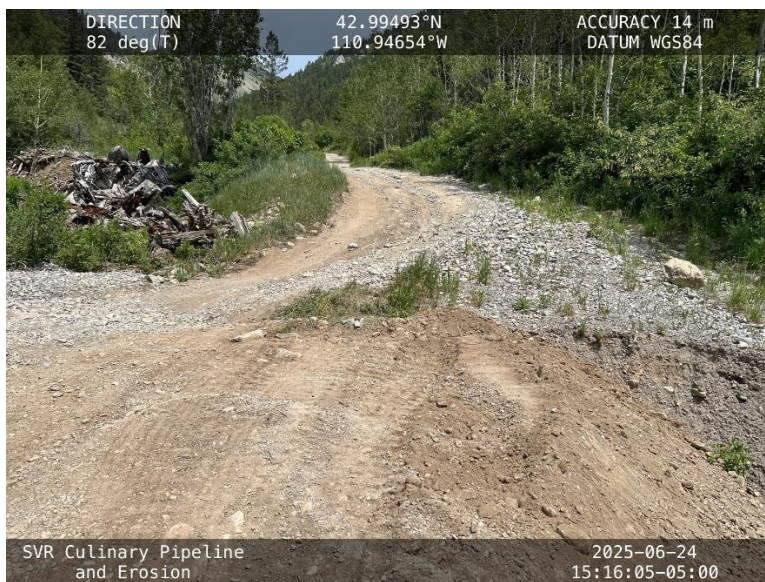
Figure D-49. Existing erosion conditions on Prater Canyon Road.
