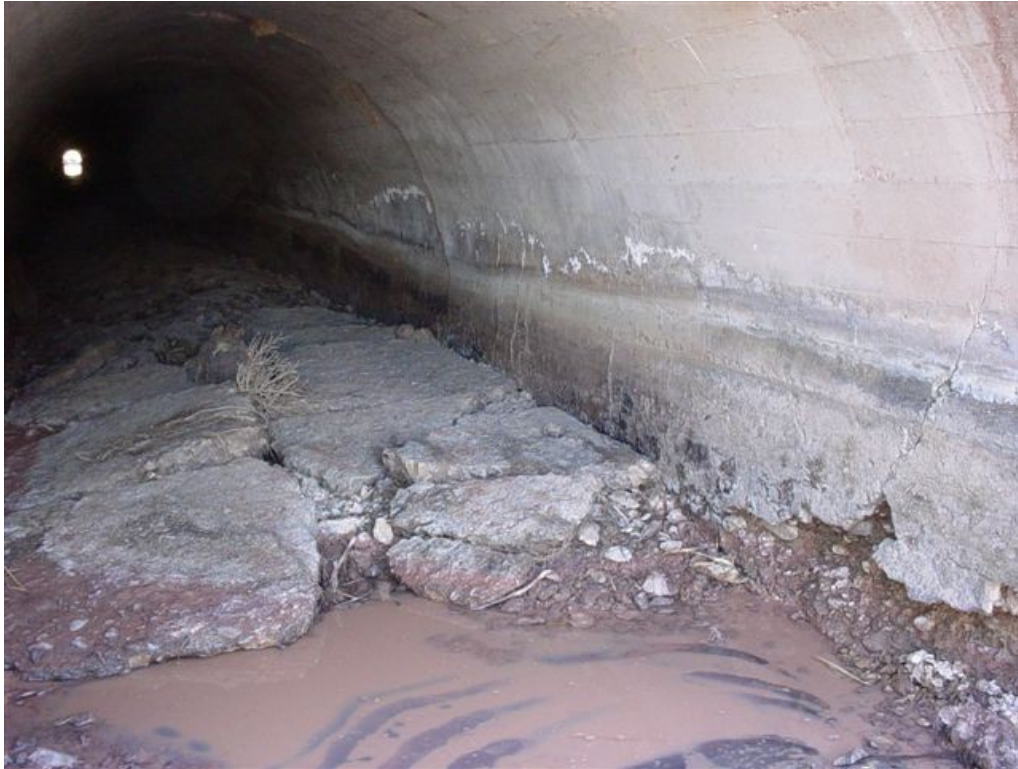
Photo 7.0.4: Missing tunnel floor.
