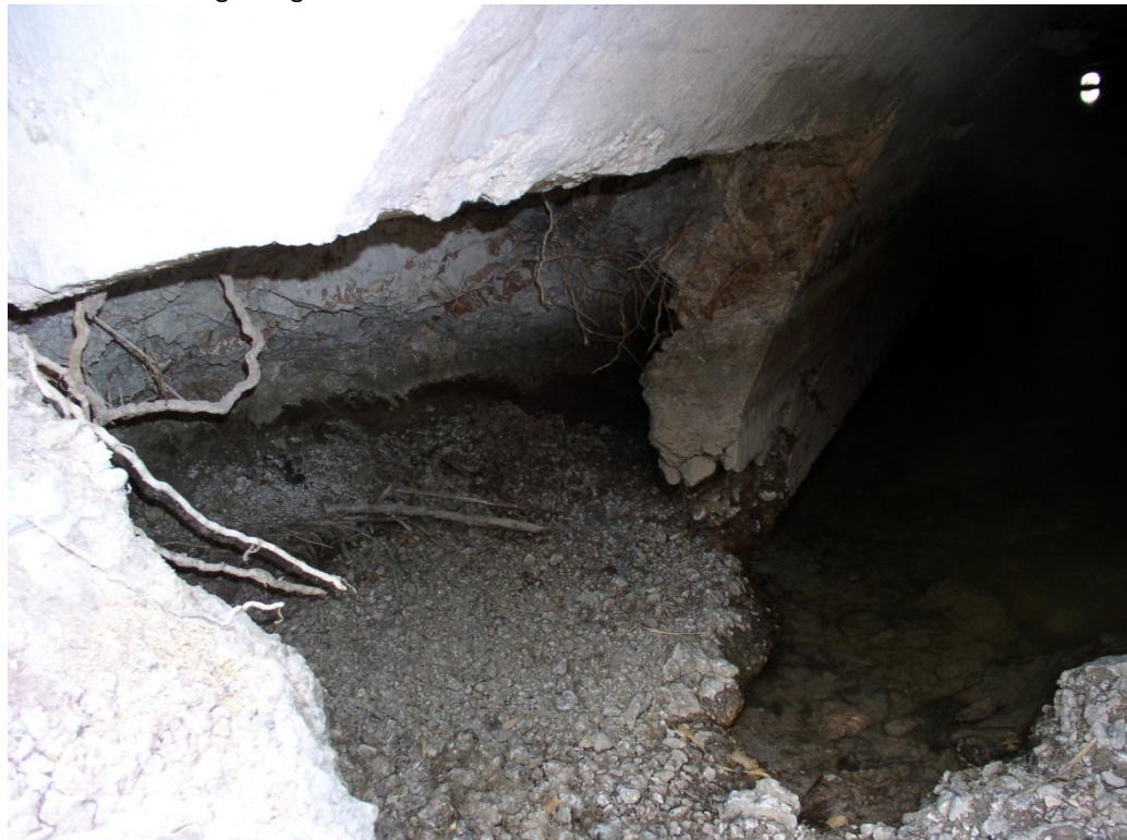
Photo 7.0.3: Missing concrete and eroded soil behind concrete.
