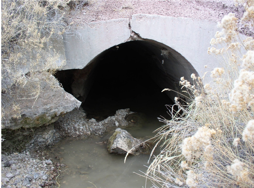
Photo 7.0.2: Degrading Concrete at tunnel outlet
