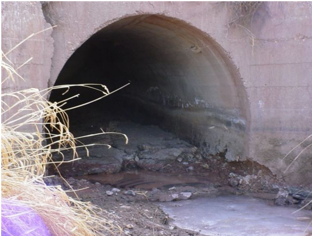
Photo 7.0.1: Degrading concrete at tunnel inlet.
