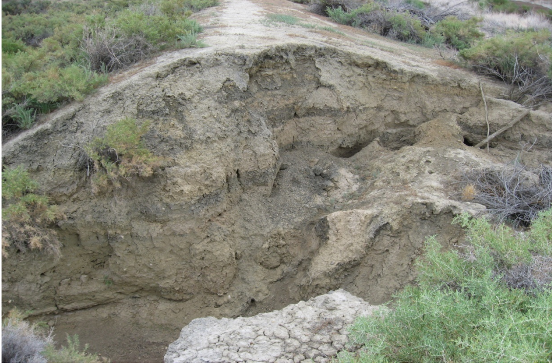
Photo 16: Collingwood Draw Middle - Break in Dam
