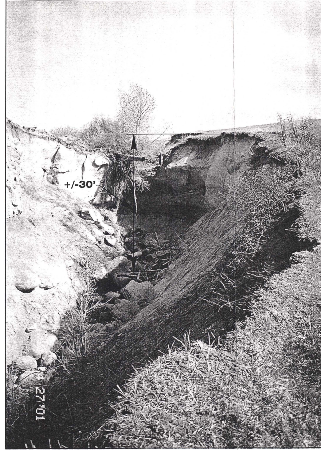
Photo B PCCDC Erosion @ 2nd Drop +/-1200' Downstream of Transbasin Diversion
