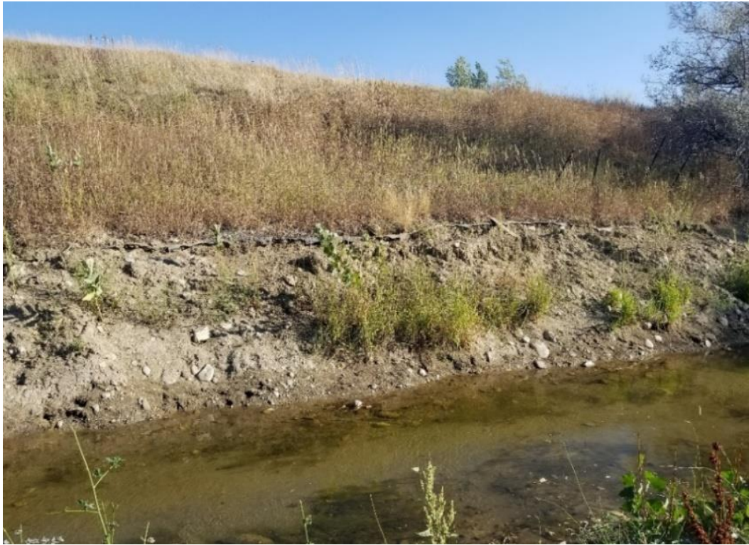
Photo 7. Dutch Flat / Taylor Ditch Adjacent to Golf Course (Geosynthetic Liner Has Been Removed).
