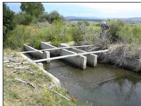
Figure 5.4. Splitter Box on Big Cottonwood Ditch.
