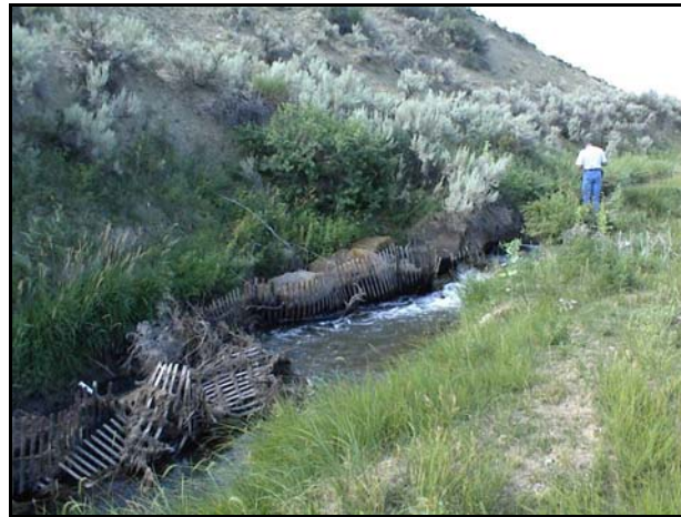
Figure 5.31 Unstable Ditch Conditions on Wise Ditch.
