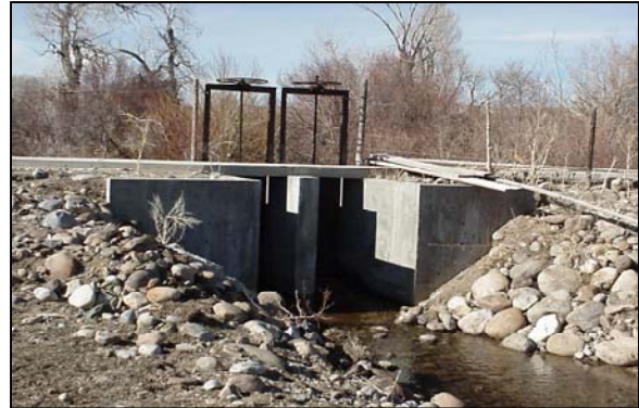
Figure 1.3 Consolidated Ditch Diversion: Example Structure Located on the North Popo Agie River.
