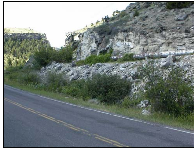
Figure 5.16 Gaylor Warnock Pipeline along CR 131.
