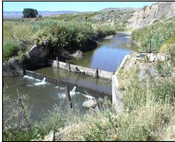
Figure 5.19 Lyons Ditch Diversion Structure on Little Popo Agie River.
