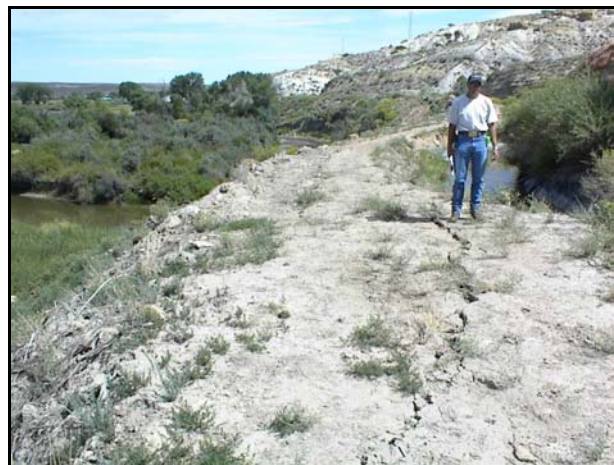
Figure 5.32 Tension Cracks in Wise Ditch Embankment.
