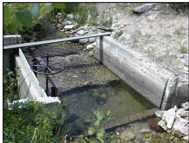
Figure 5.17 Sediment Trap on Gaylor Warnock Ditch.
