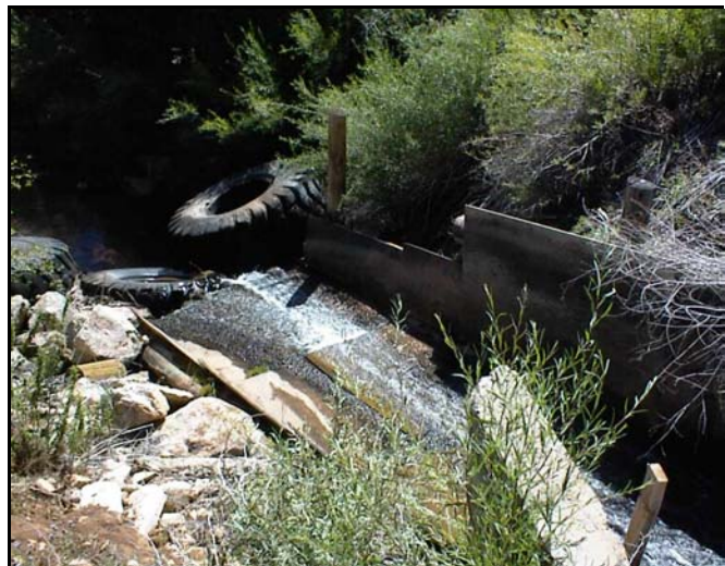
Figure 5. 14 Turnout and Drop Structure in Poor Condition on Enterprise Ditch.
