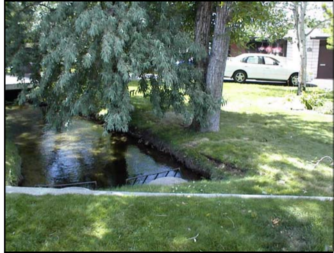
Figure 5.6 Cemetery Ditch in Subdivision Showing Example of Driveway Culvert Restricting Conveyance.
