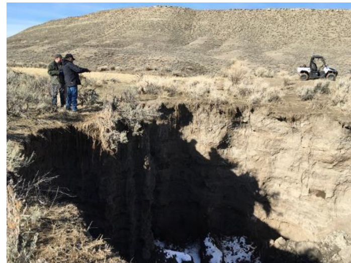
Headcut 2 looking downstream
