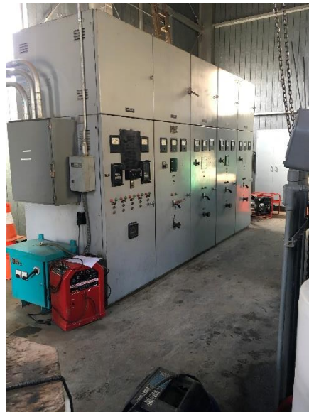
Level II Project: Lucerne Pump Motor Control Center
