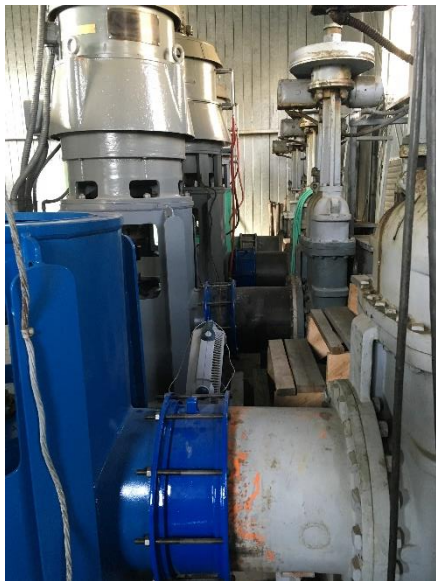
Level II Project: Lucerne Pumps
