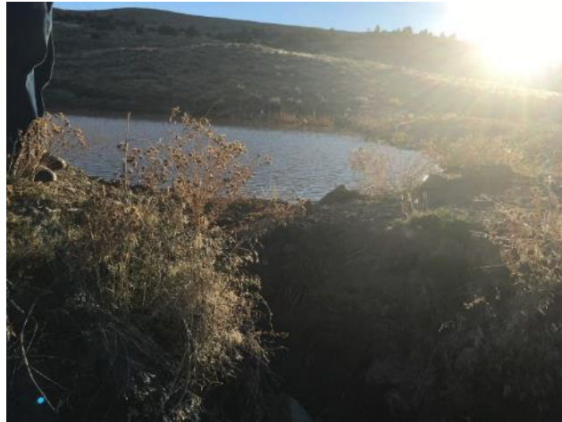
URI-007 Spillway Erosion
