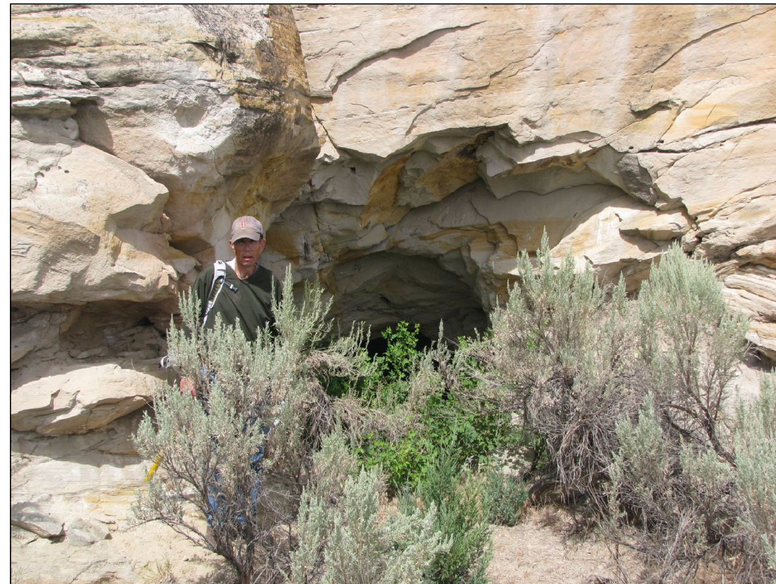
B SMALL CAVE AT BASE OF LEFT ABUTMENT
