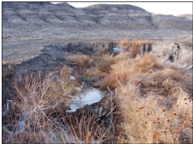
Figure 3.63 Erosion Near Tail End of the Anita Ditch
