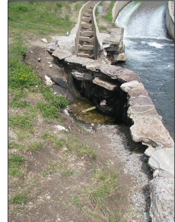
E EROSION DOWNSTREAM OF FISH LADDER
