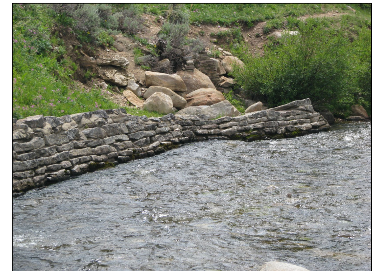
F EROSION DOWNSTREAM OF SPILLWAY ALONG LEFT BANK
