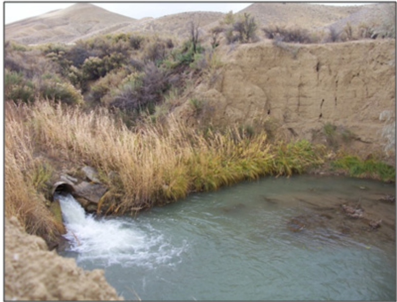
Figure 3.64 Outlet of Drop Structure in Poor Condition on the Avent Ditch
