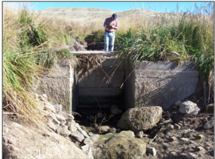
Figure 3.66 Check Structure on Highland Ditch
