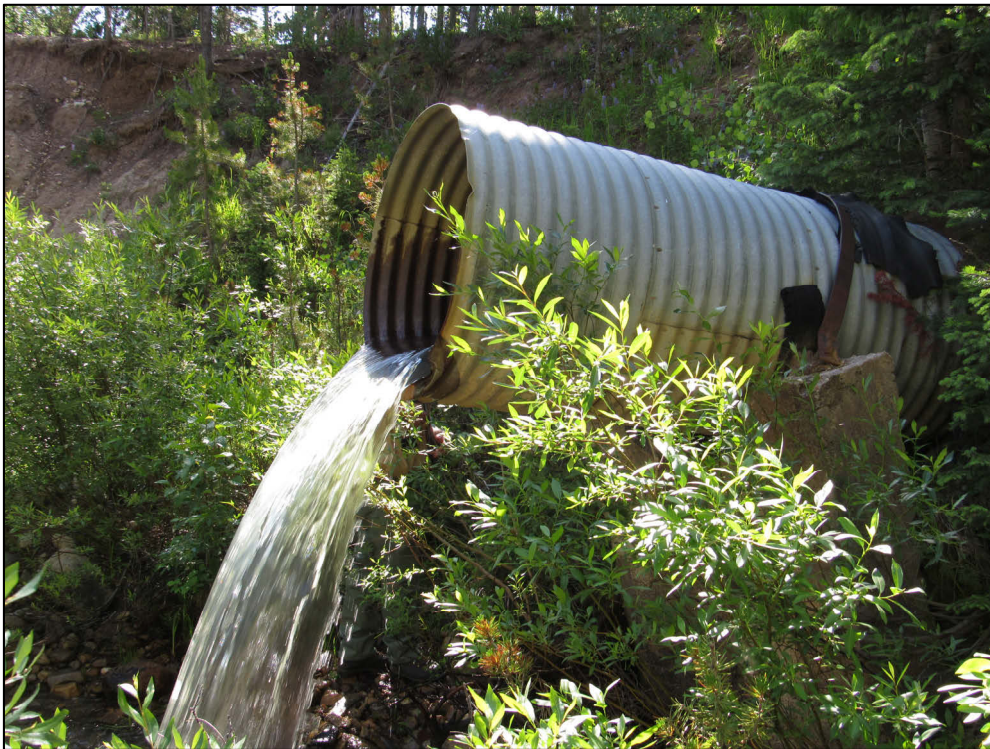
Figure 4.3-16 Failing drop structure on the Highline No. 1 ditch. Note the leaning concrete support wall and slope of the CMP indicating failure of internal welded joint(s).
