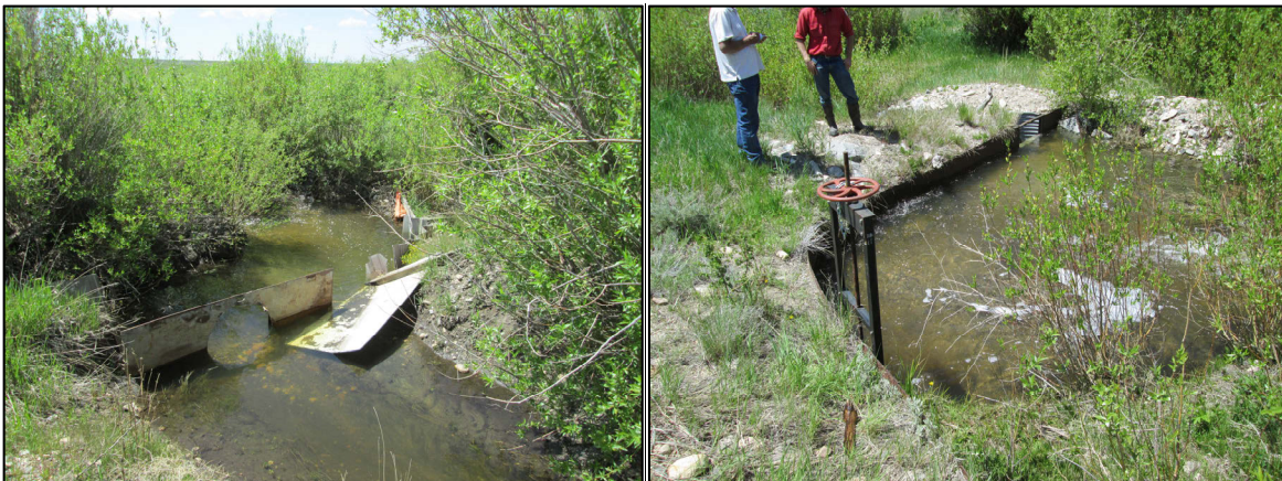
Figure 4.3-9. Existing North Meadow Ditch Headgate (left) and recently constructed headgate on adjacent ditch (right). Both structures are located on South Fork Lake Creek.
