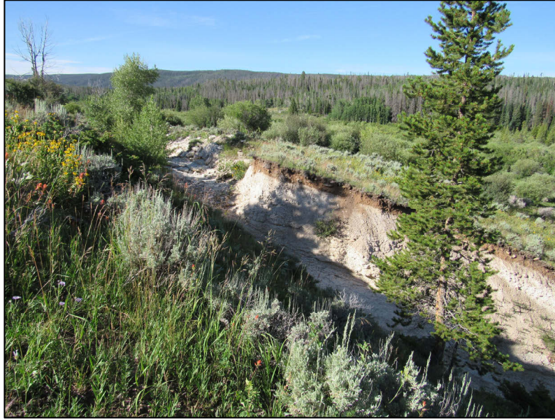
Figure 3.3-6 Brush Creek Supply Ditch erosional feature.
