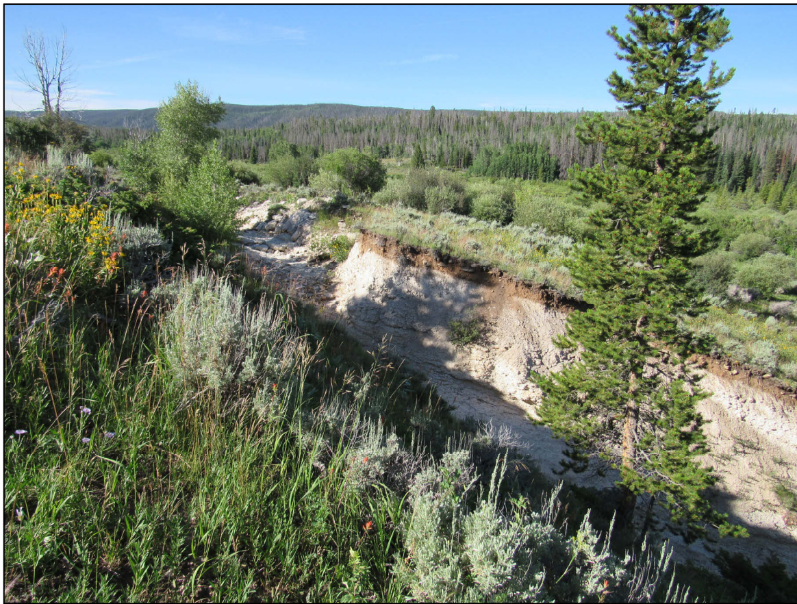
Figure 4.3-14. Erosional feature on South Brush Creek Supply Ditch.
