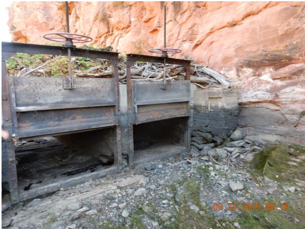
Figure 3.28. LaPrele Main Canal Diversion Headgate Structure and Slide Gates.
