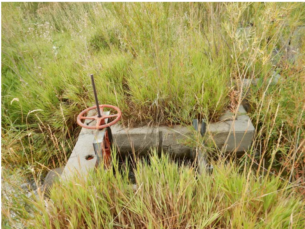
Figure 3.46. View of a Lateral No. 9A Sublateral Headgate Structure.
