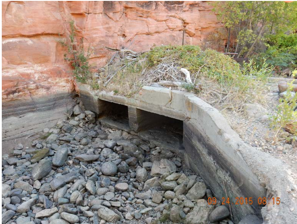
Figure 3.29. Broken Concrete (Middle) on the LaPrele Main Canal Diversion Headgate Structure.
