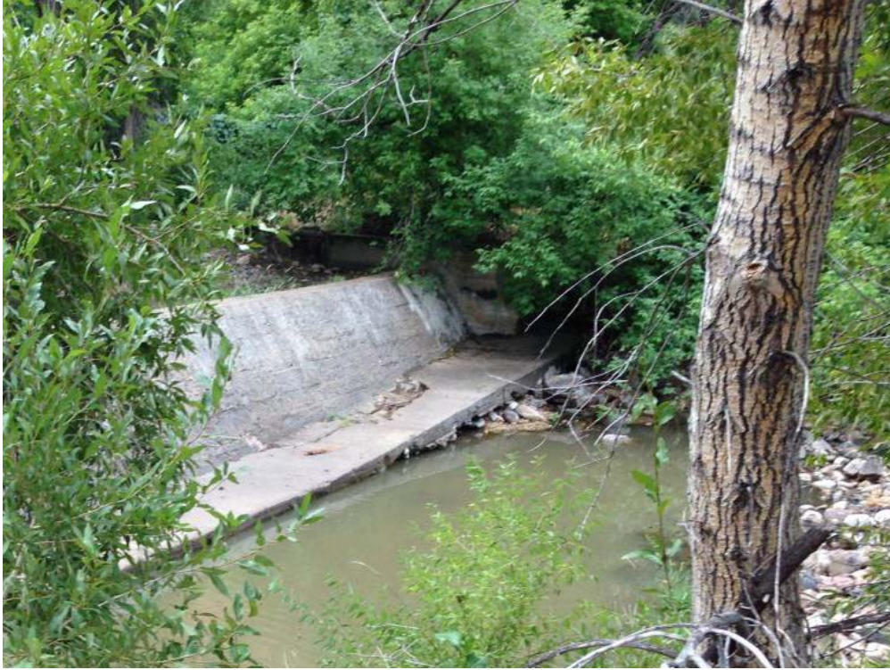
Figure 3.27. LaPrele Creek Bed Scoured Below the Main Canal Diversion Weir Apron (Right Middle).
