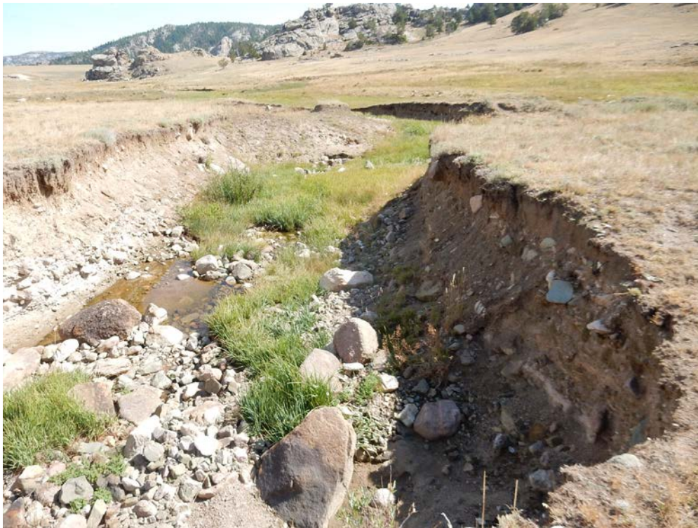
Figure 3.121. Headcut on the Earthen Spillway of Westfork No. 1 Reservoir (Blue Downey).
