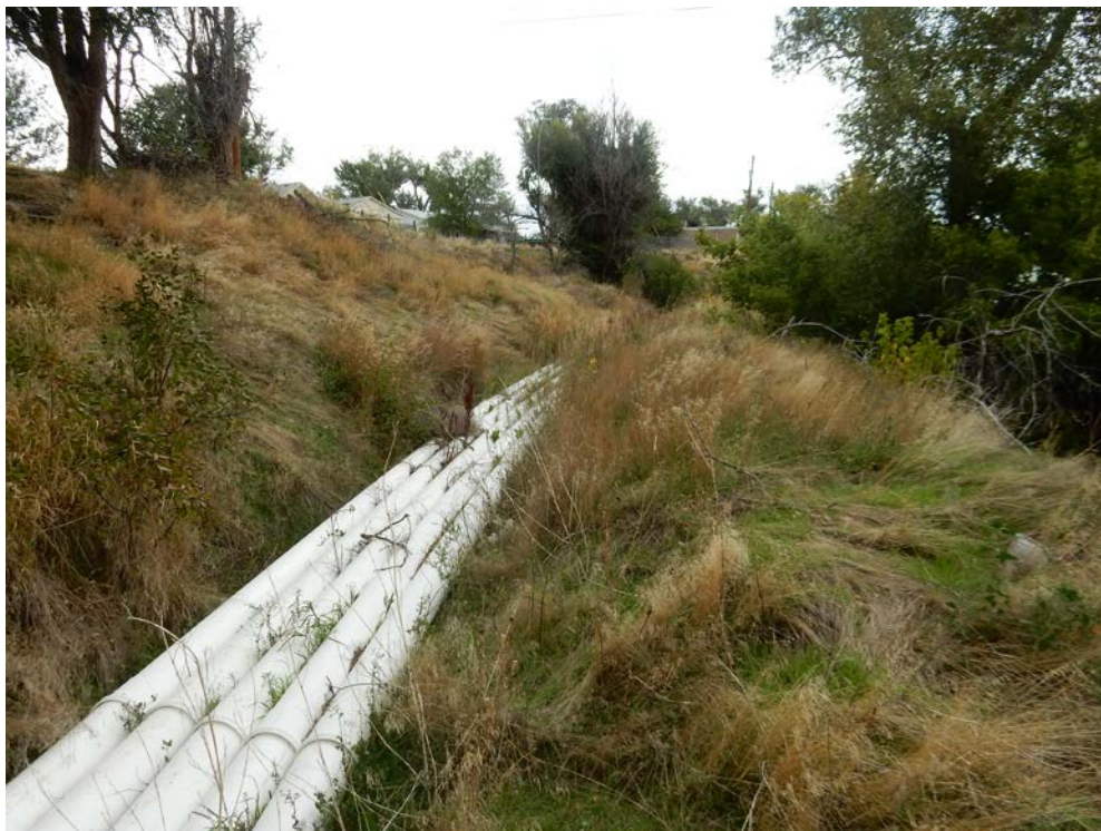
Figure 3.63. Carey No. 2 Ditch With 10-Inch Plastic Irrigation Pipeline Laid on the Bottom.
