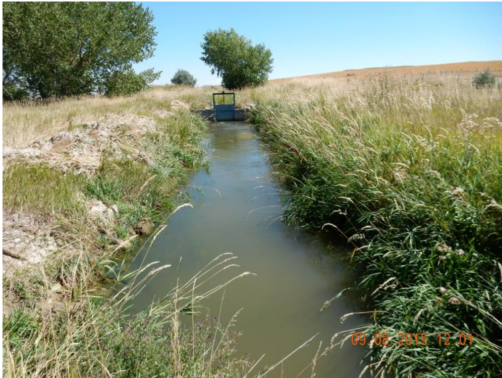
Figure 3.36. Lateral No. 1 From the Main Canal Near the Division Box for Laterals No. 1 and No. 2.
