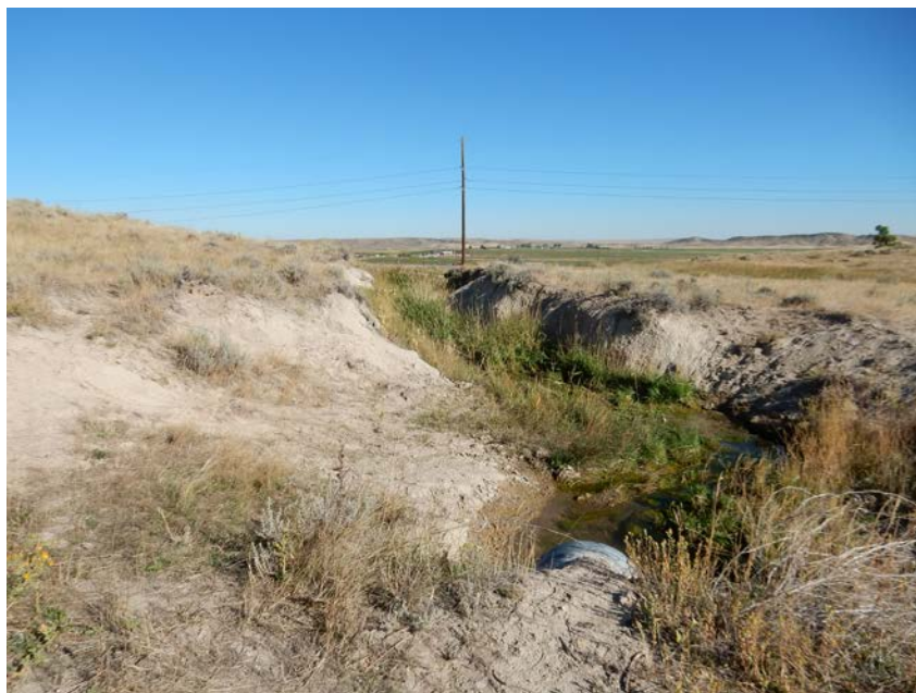
Figure 3.50. Downstream View of Lateral No. 2A Sublateral From the Headgate on Lateral No. 2A.
