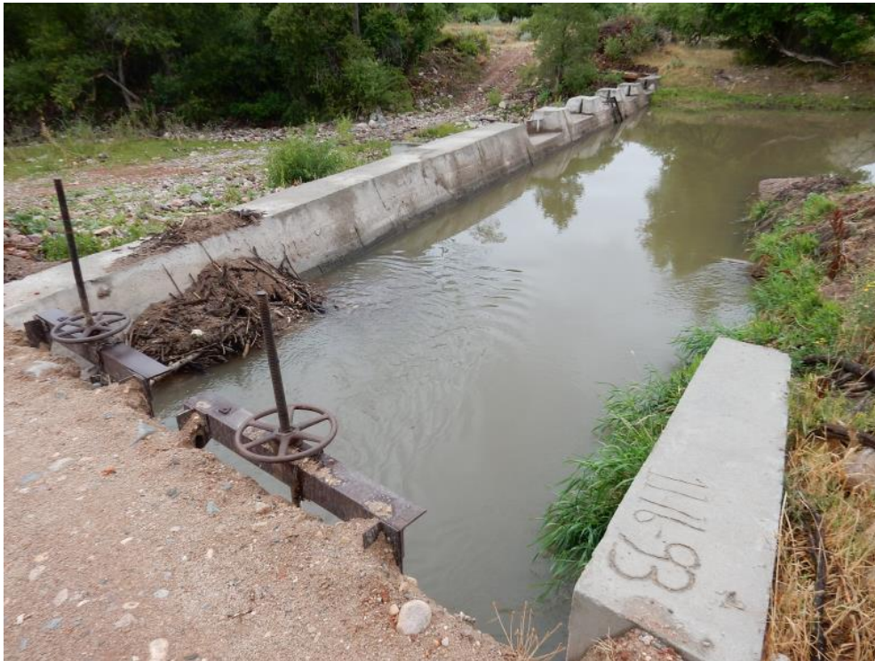
Figure 3.43. LaPrele Westside Canal Diversion Headgate Structure and Slide Gates.
