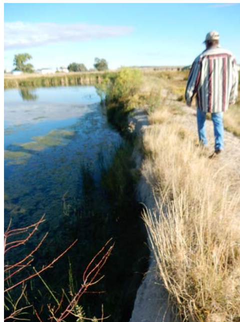
Figure 3.123. View of the Embankment Erosion on the Larime No. 1 Reservoir.
