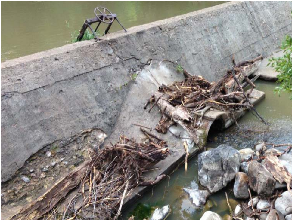
Figure 3.26. Concrete Spalling (Lower Left), Crack (Middle, Below Slide Gate Handwheel), and Broken Apron (Upper Right) on the LaPrele Main Canal Diversion Weir.
