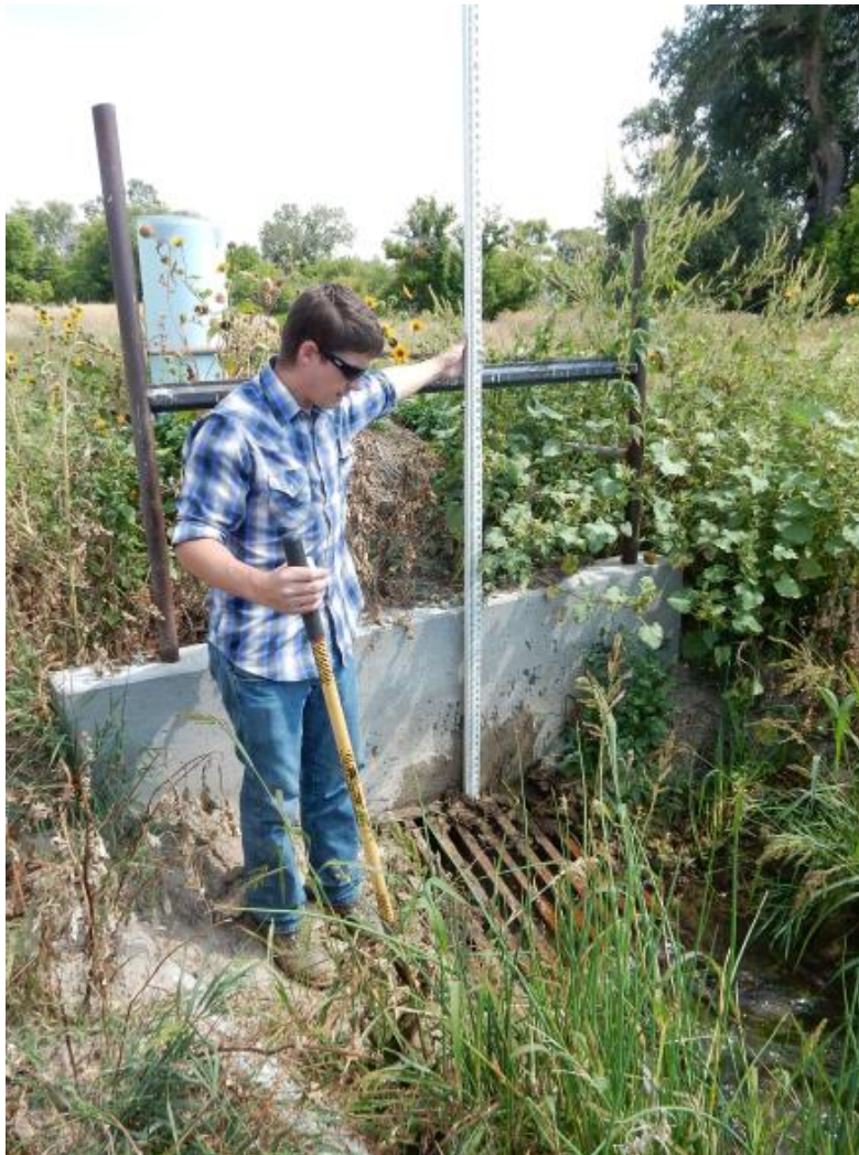
Figure 3.52. Pipe Inlet on the Walker No. 3 Ditch. The open ditch upstream from this point experiences periodic damage from cattle.
