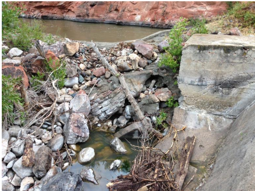
Figure 3.30. Scour of the LaPrele Main Canal Berm (Middle) Behind the Headgate Structure (Right).
