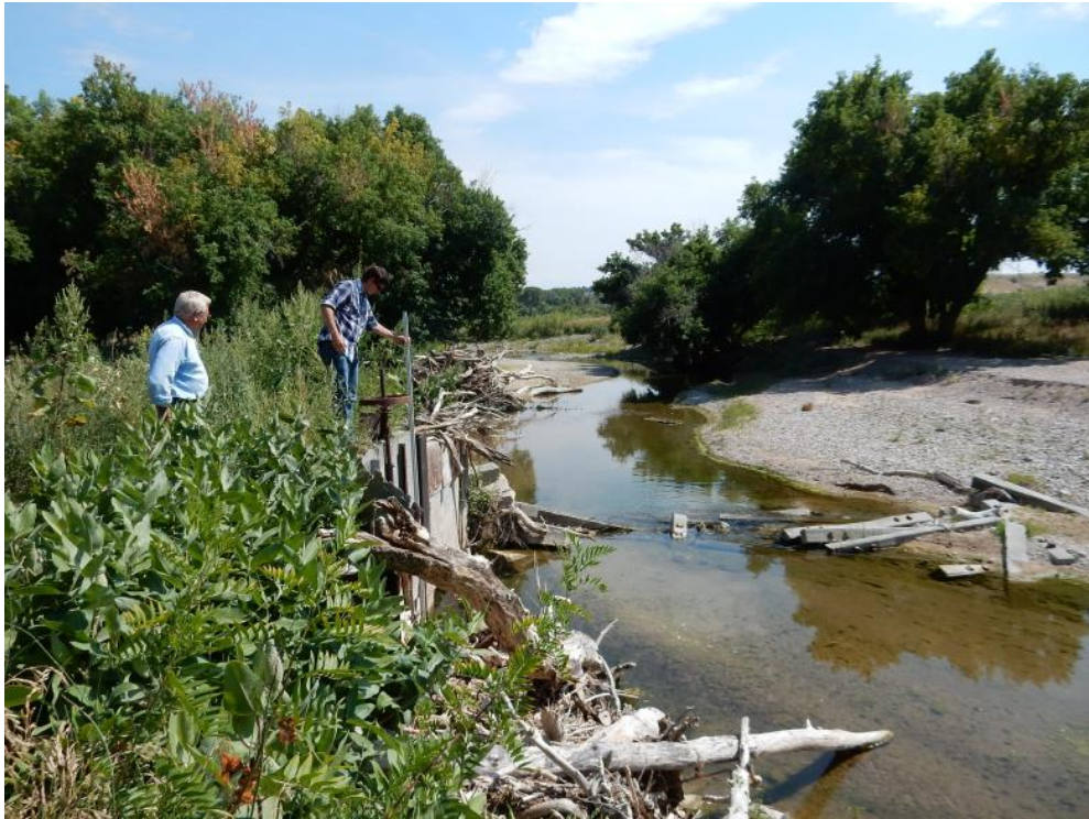
Figure 3.53. Hoffman Ditch Diversion (Left Middle).
