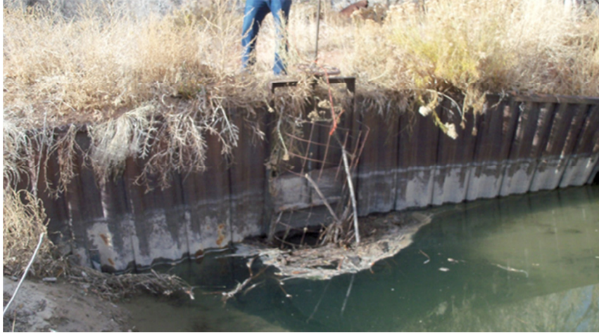
Figure 4.1. Garrett Ranch Headgate on Bates Creek.
