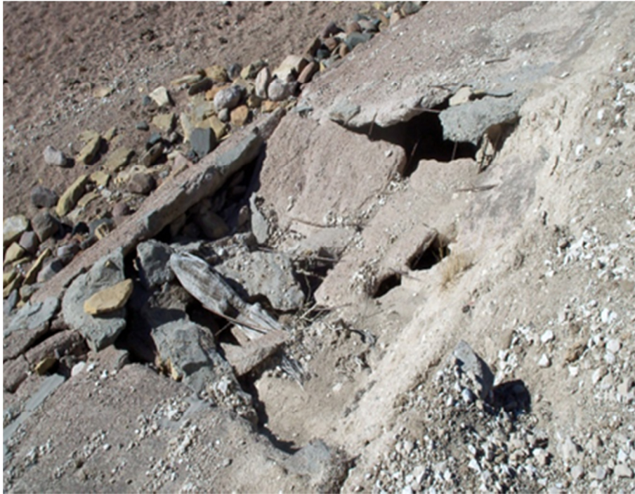
Figure 4.41. Concrete Slope Revetment Failure on Dam.
