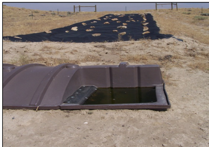
Figure 4.34. An Example of an Installed Wildlife Guzzler System.
