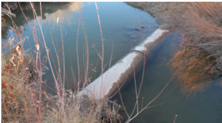
Figure 4.2. Siphon Exposed by Channel Degradation on Bates Creek.
