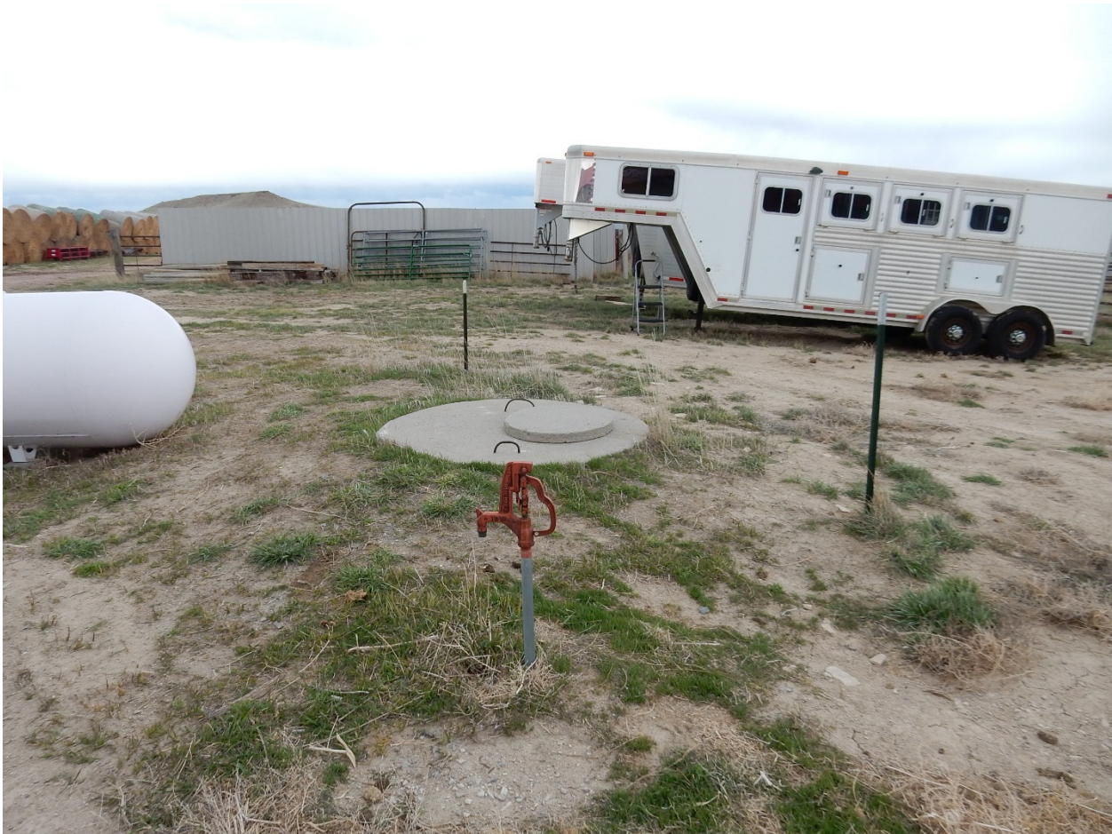
Figure 4.32. Existing Raezer #1 Well and Pump.
