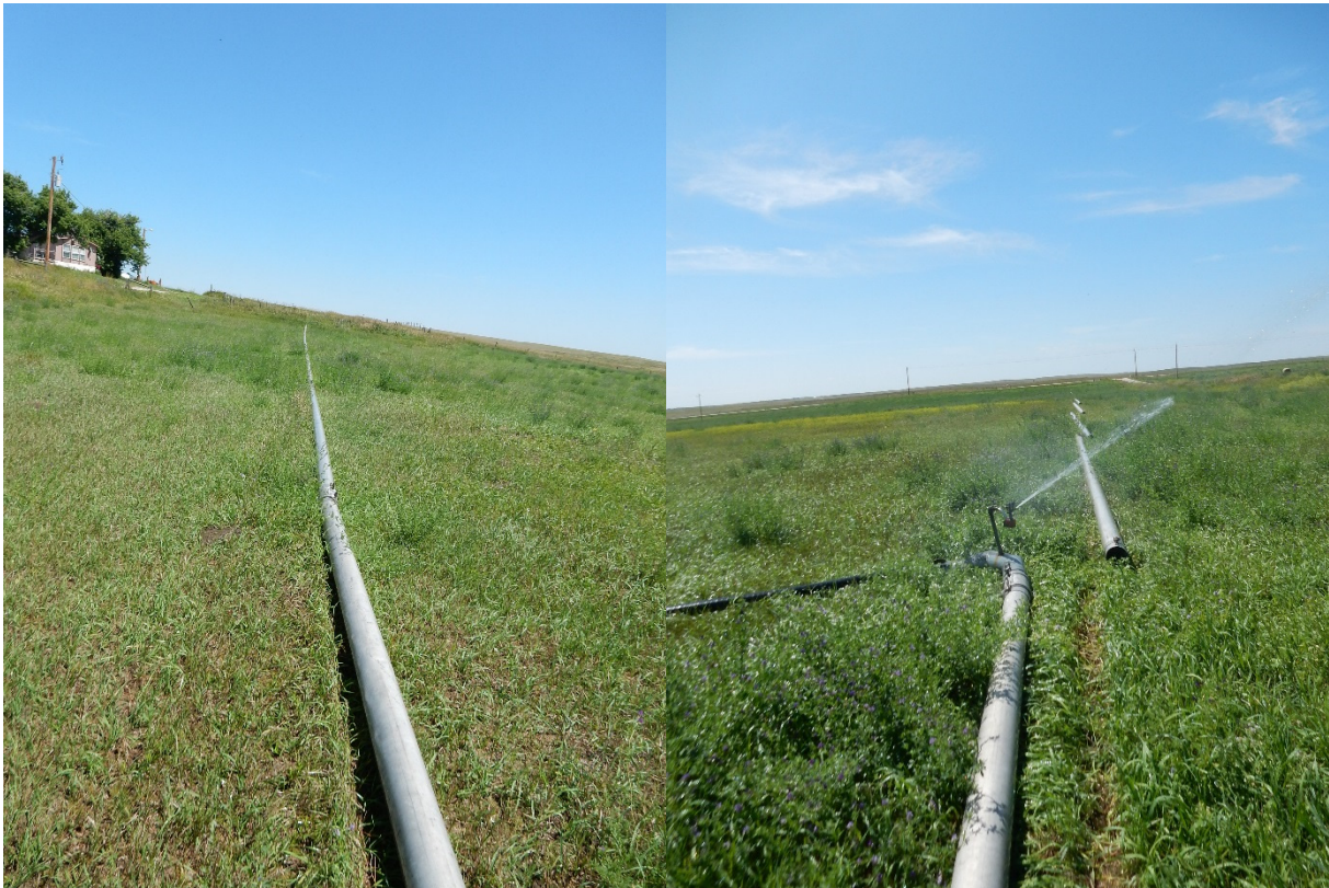
Figure 4.11. Existing Above Ground Mainline Supplied by The Ladwig No. 2 Well.
