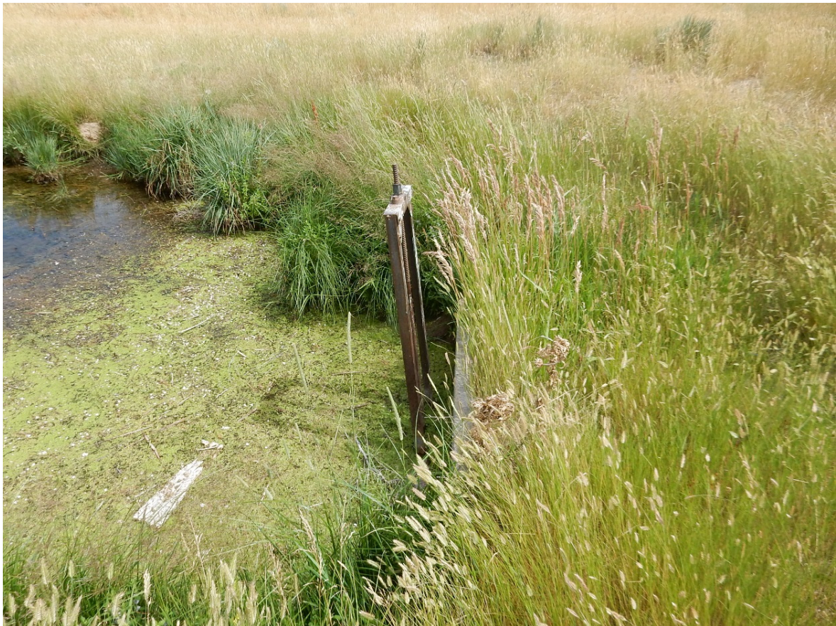
Figure 4.3. Headgate Structure on Hoblit Reservoir for Reynolds No. 1 and Reynolds No. 2 Ditches.
