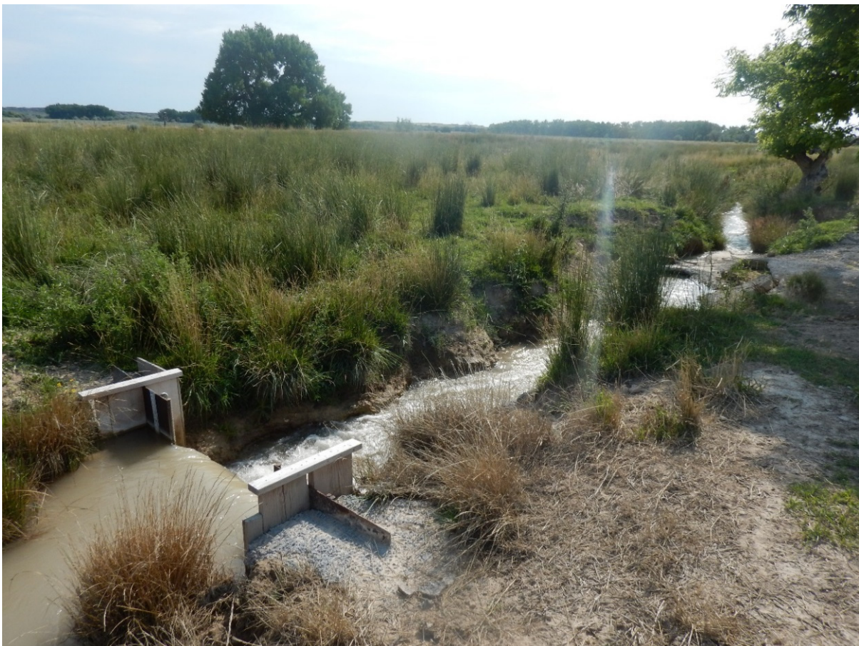
Figure 4.17. Weir and Downstream Failed Concrete Diversion on Box Elder Creek for Glomill Ditch.
