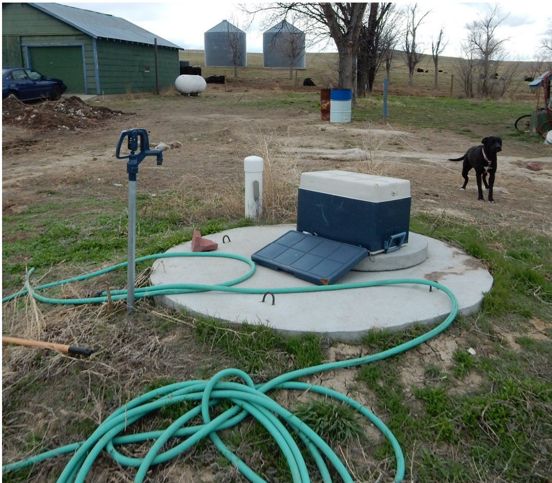
Figure 4.34. Existing Raezer #2 Well and Pump.
