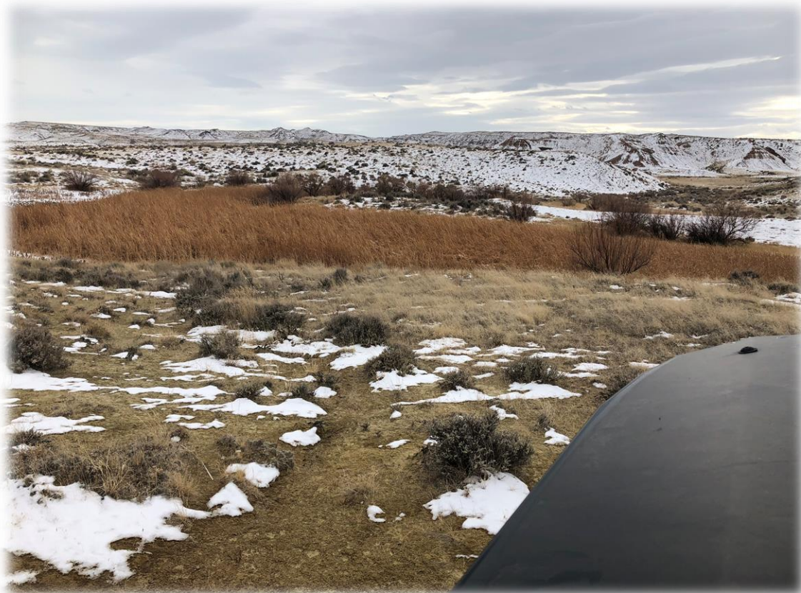
Figure 90: Silted in and vegetated silt dam.
