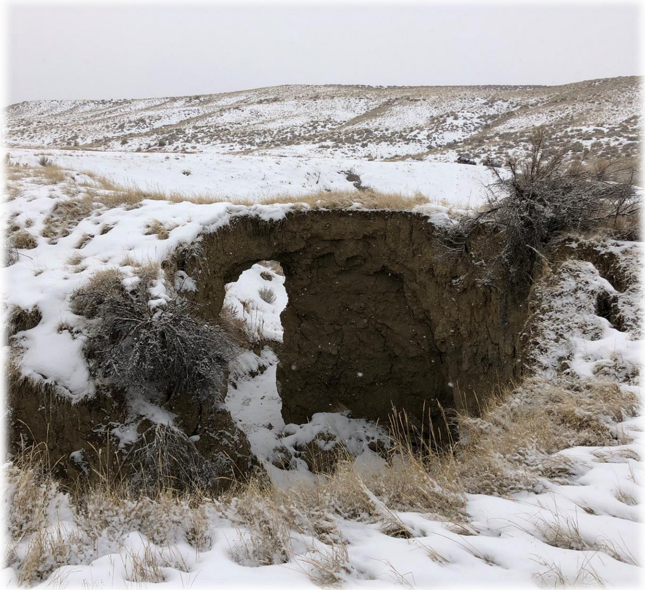
Figure 91: Eroded silt dam.
