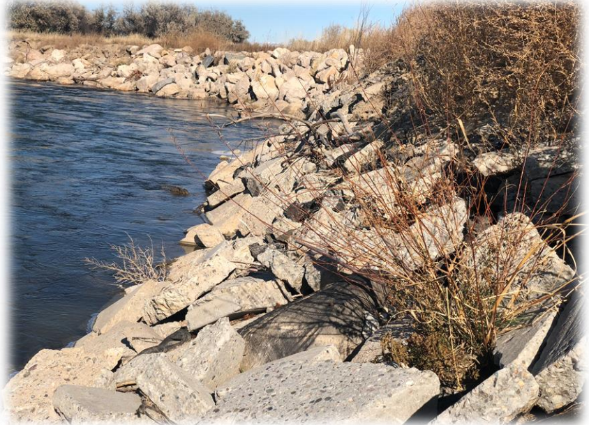
Figure 29: Revegetated and reconstructed riverbank in proximity to erosion that uncovered sewer main.
