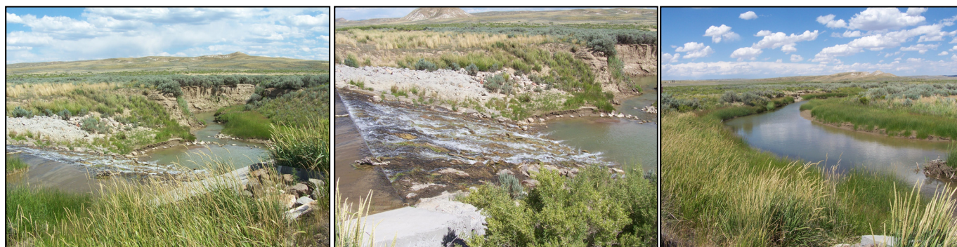
Figure 3.6-9 Muddy Creek Gradient Restoration Structure. From Left to right, view downstream, view of the structure, and view upstream.
