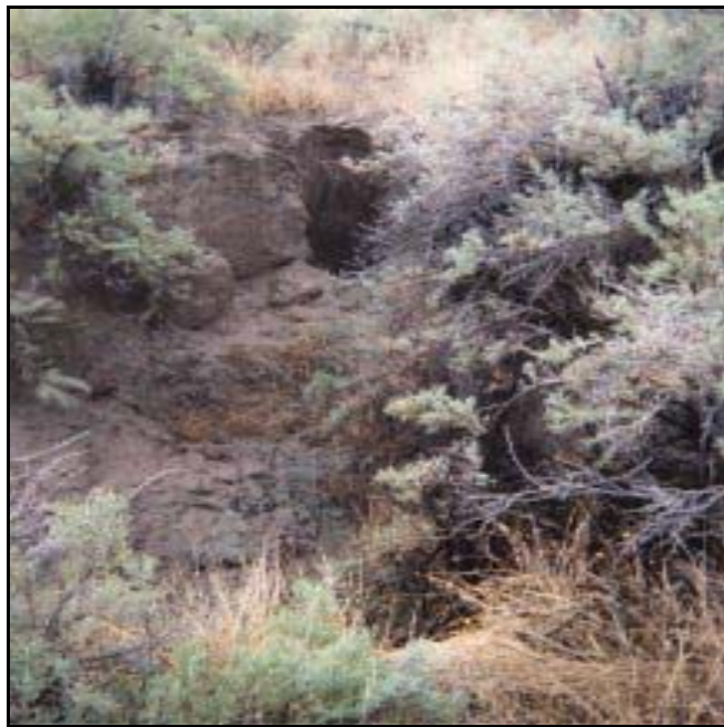
Photograph 10. Water from the tributary enters the Kirby Creek gully through the ‘pipe,’ the black hole in the ground (upper center of photo) from the tributary bed level to the vertical bank of the creek
