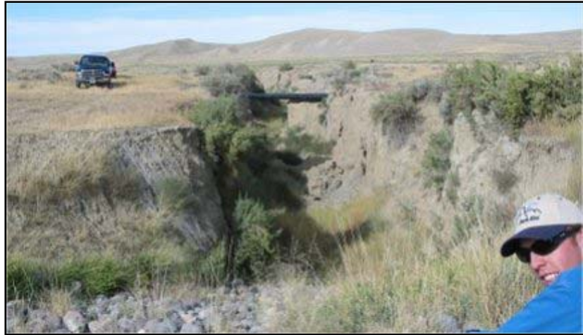
Photograph 16. View of gully looking downstream. There is an oil pipeline suspended across the gully. This is another Rosgen Type G stream for a short ways downstream.
