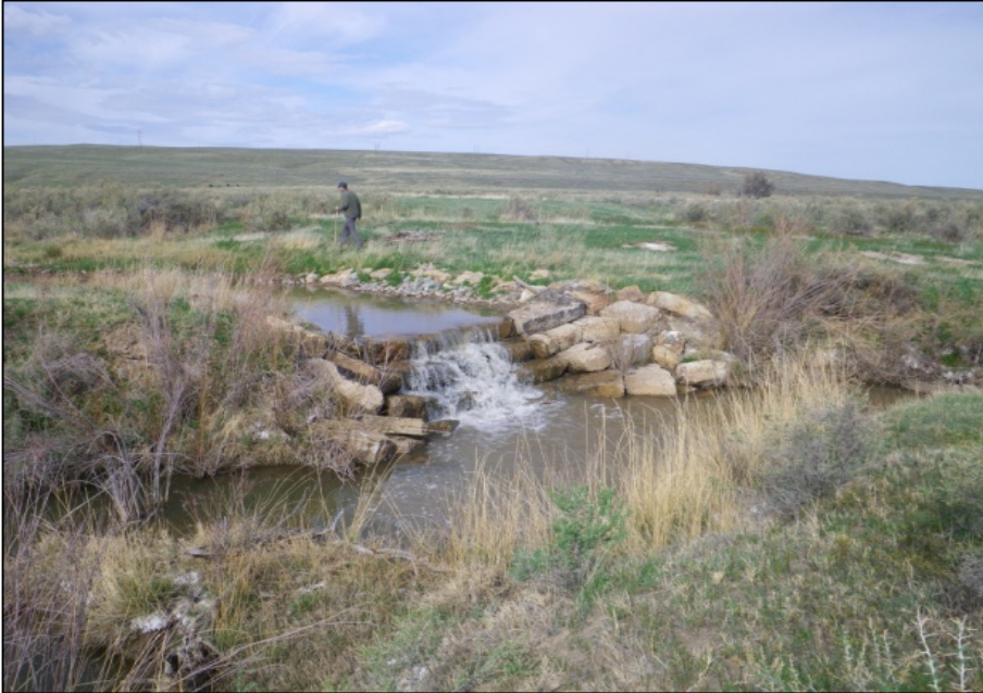
Figure 3.50. Drop structure located at downstream end of Lucy Moore Project.
