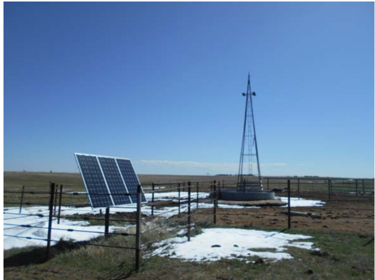
Figure 1.2-2 Typical SWPP Project: Failed Windmill Replaced with Solar Pump and Platform.
