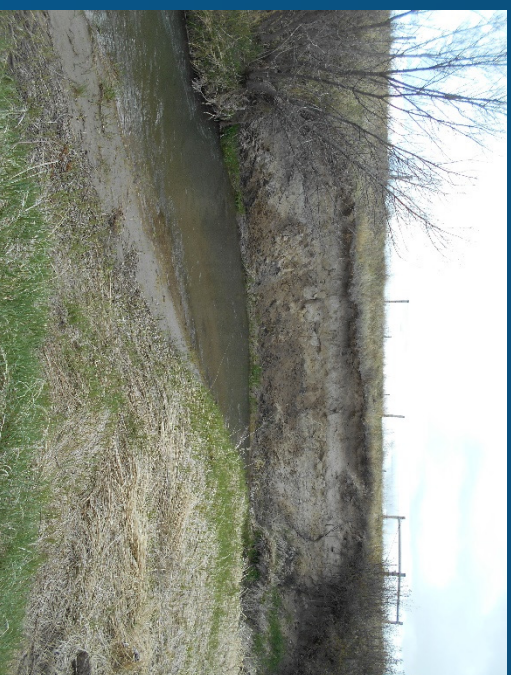
Bank Erosion: Horse Creek
