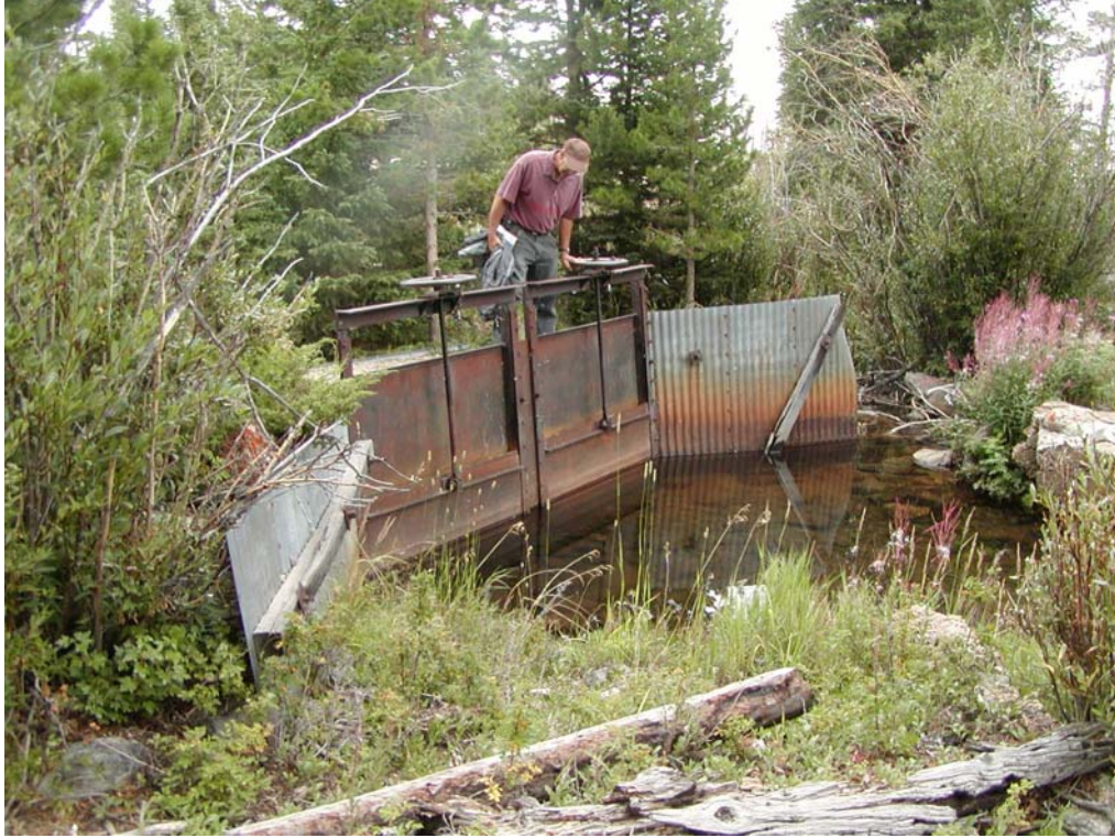
4 Lakes and French Creek Diversion – Headgate
