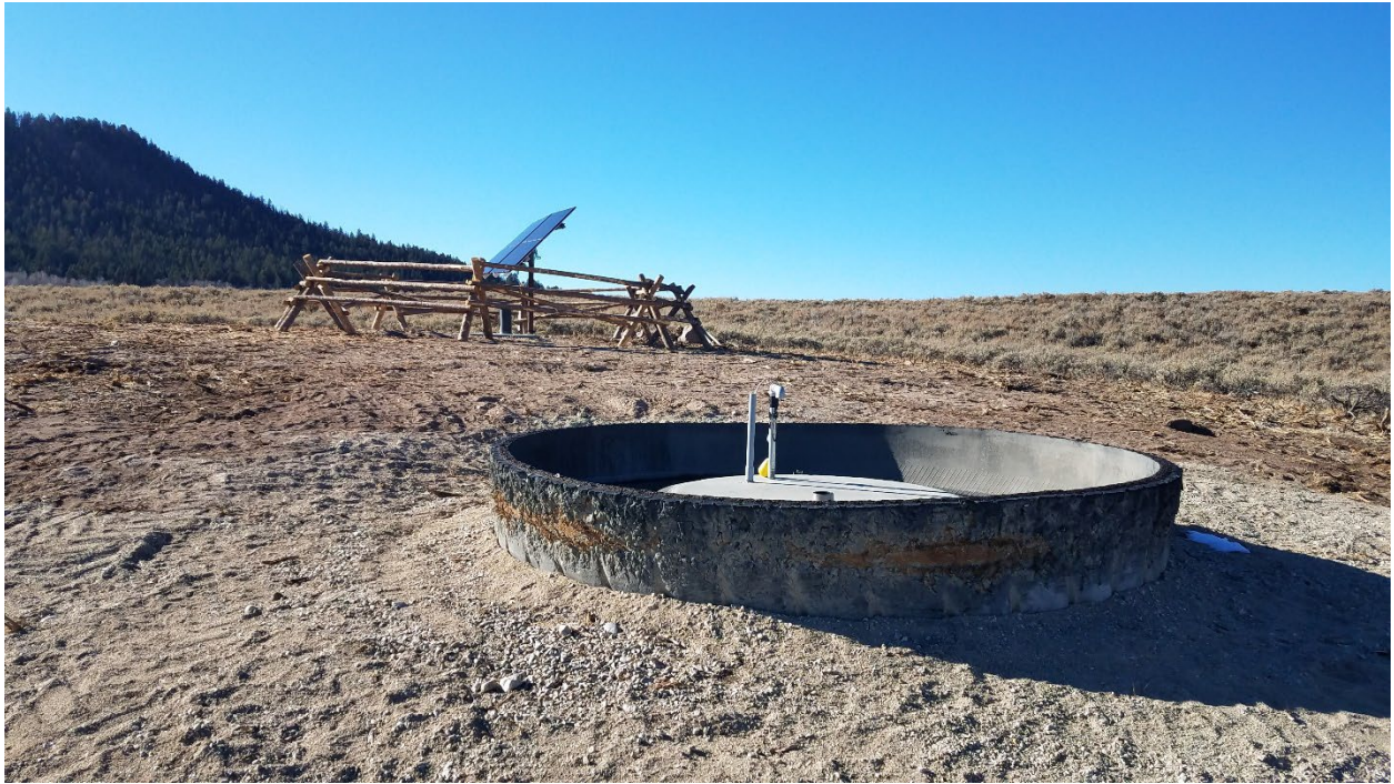
Example 7: Stock water well, solar platform, and stock water tank project
