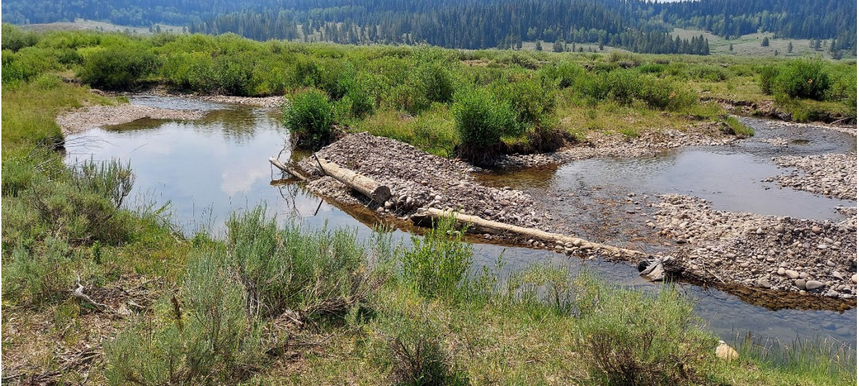
Example 3: Diversion structure to be reconstructed by use of cross vane (Account II – Diversion Structures)
