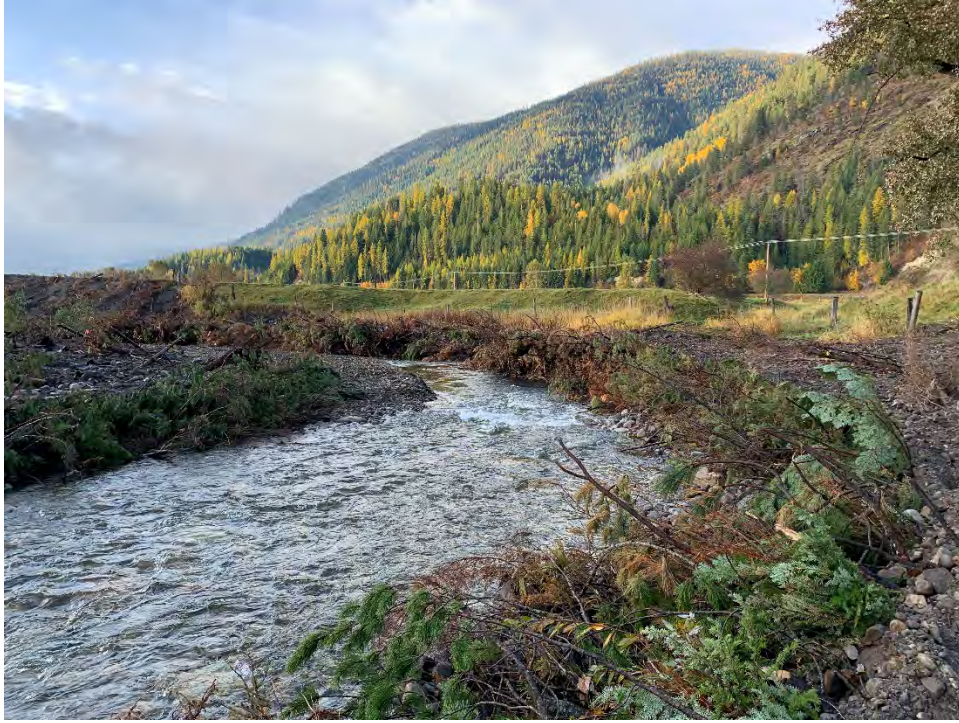
Photo 7: Vegetated brush bank structure for bank stability and improved fish habitat, Ball Creek, MT.
