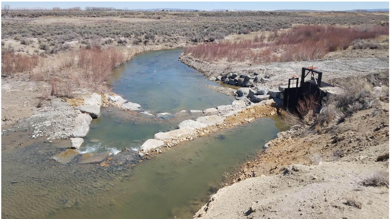
Example 8: Diversion structure and head gate rehabilitation project (Big Sandy Watershed Study)
