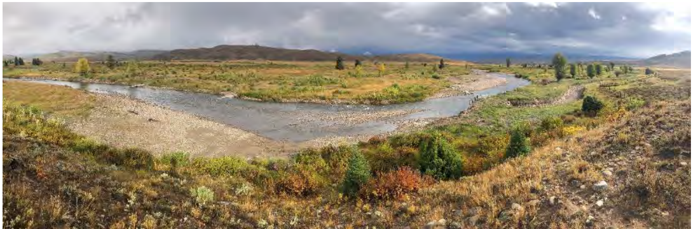
Photo 4: Panoramic photo of diversion site showing j-hooks and bankfull bench upstream, new headgates and enlarged supply ditch, and cross-vane irrigation diversion structure installed in Phase 1.
