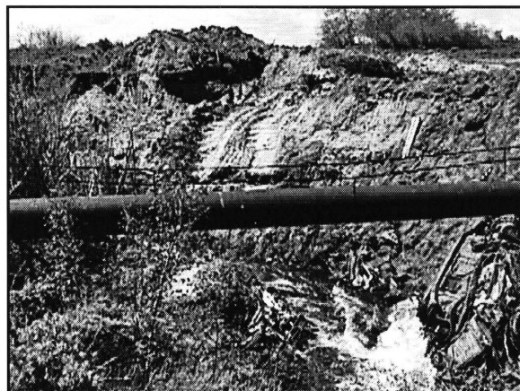
Figure 1.5 Degradation of Wiant Ditch at Ryan Foreman Pipeline Crossing.
