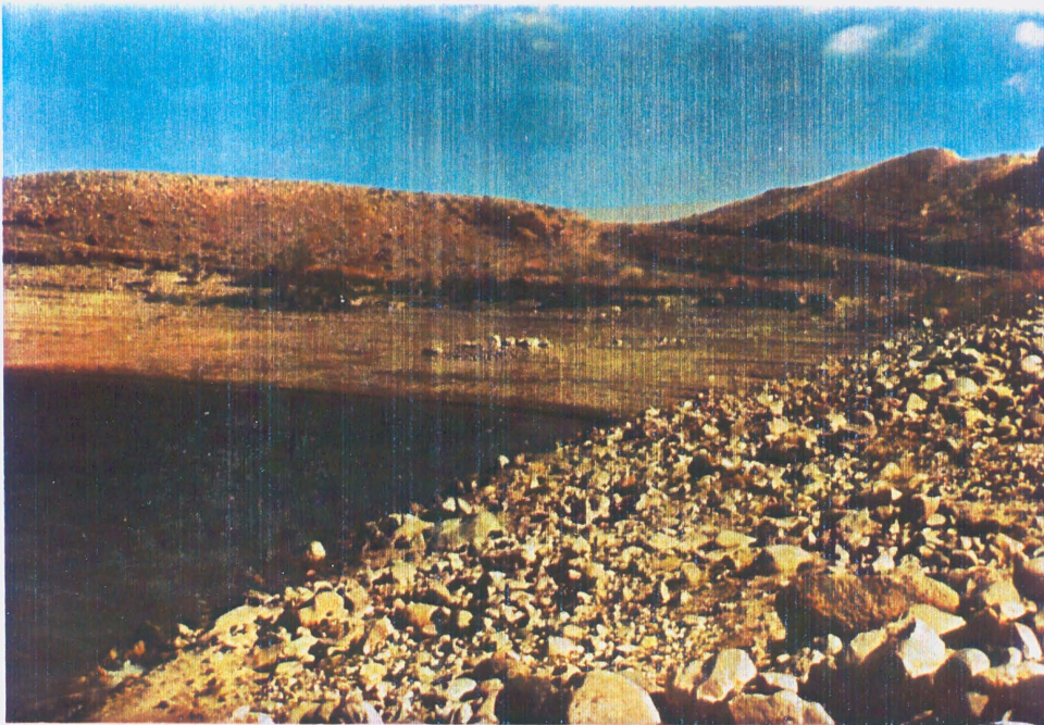
LEFT (EAST) ABUTMENT RIPRAP - SOUTH EMBANKMENT MUDDY GUARD NO. 2 RESERVOIR PROJECT NO. 7
