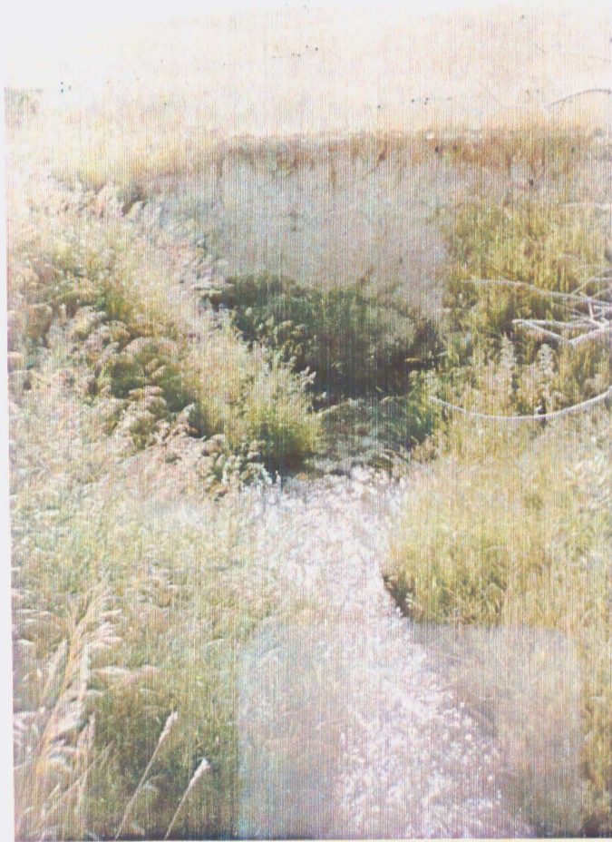
EROSION: ROGERS-ESPY-FRALEY-BENSON DITCH PROJECT NO. 1 - STA 45+12
