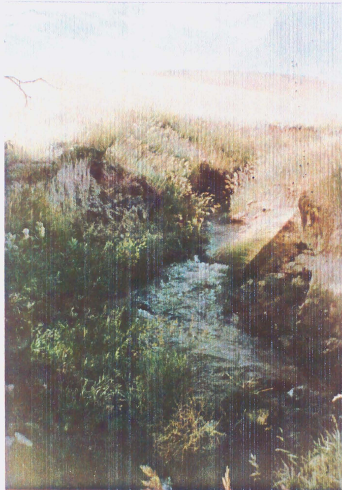
EROSION: ROGERS-ESPY-FRALEY-BENSON DITCH PROJECT NO. 1 - STA 45+12
