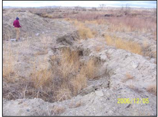
Figure 2.5-9 Severe Gully Erosion at Wales Ditch
