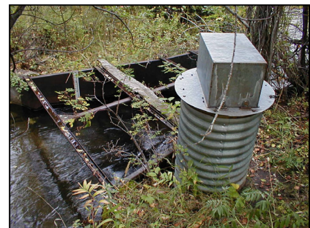
Piney & Cruse flume, recorder, primary diversion, North Fork of Piney Creek
