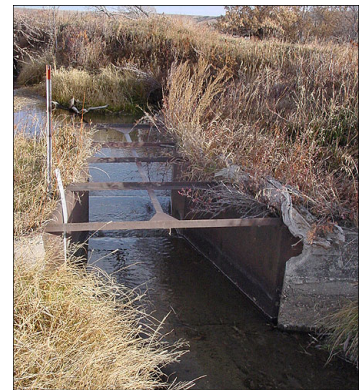
Hopkins Ditch flume
