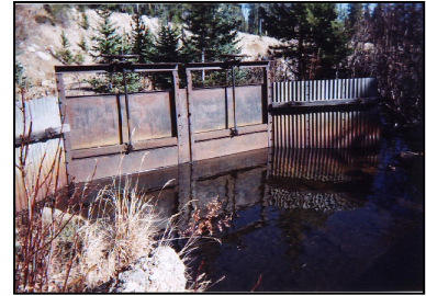
Four Lakes & French Creek headgates
