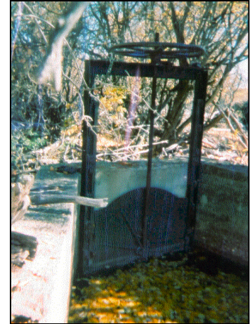
Penrose Ditch at French Creek headgate
