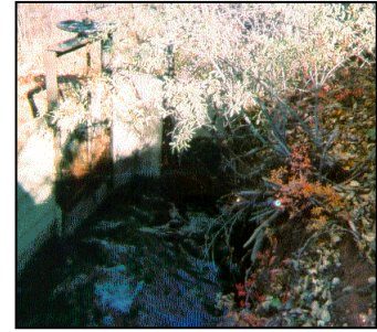
Mowry Basin headgate
