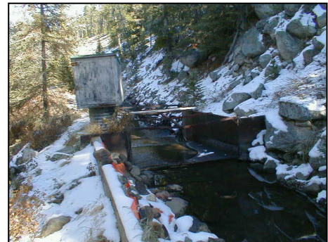
Rock Creek & South Piney flume and gage
