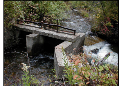
Piney to Little Piney headgate
