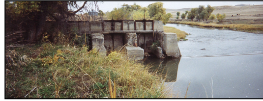
Pratt & Ferris No. 3 headgate
