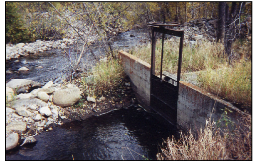
Six Mile headgate
