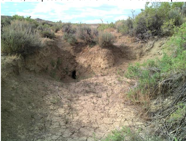
Head cut in spillway
