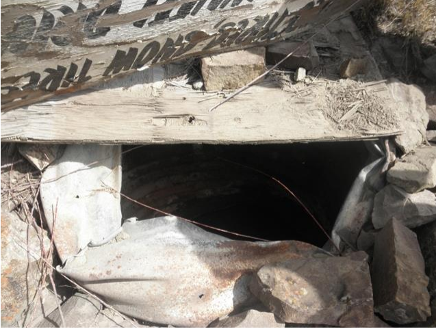
Bridger Well No. 13 collection box
