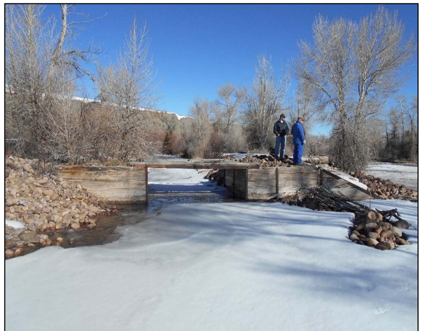
Figure 3.2-7 Bridger Butte Diversion Structure.
