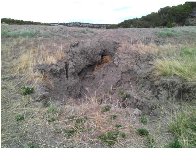
Breach in Bridger No. 10 Pond embankment
