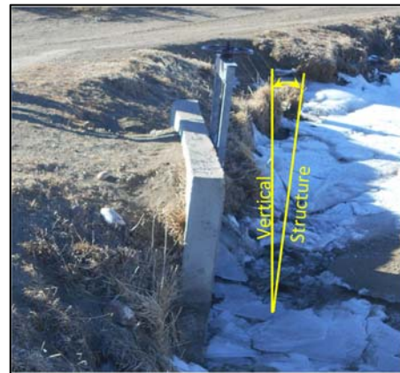
Figure 3.2-5. Failing Farm Turnout Headgate on Bridger Butte Canal.
