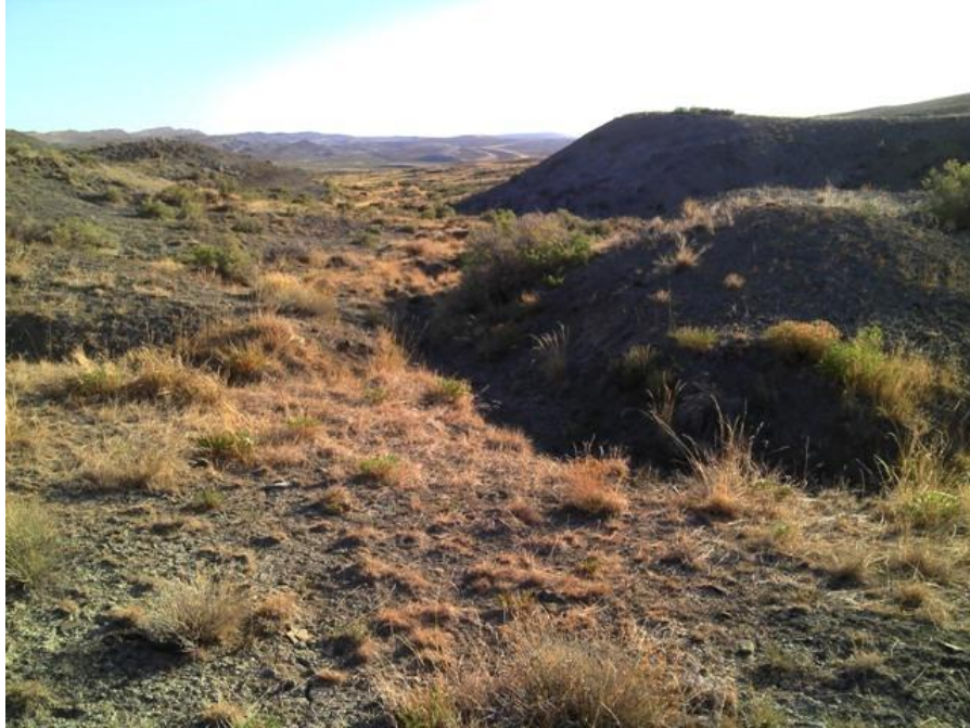
Cumberland No. 9 breach and head-cut in existing pond embankment
