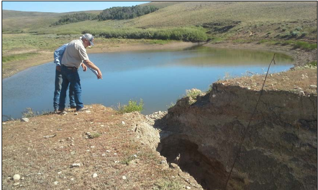
Figure 3.3-14 Reservoir Embankment Failure.
