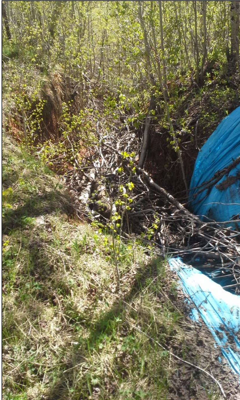
Figure 3.5-7 Davis No. 2 Reservoir outlet channel incision.
