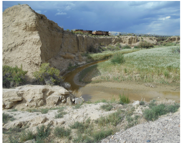
Figure 4.2-29 Active Channel Degradation: Bitter Creek.
