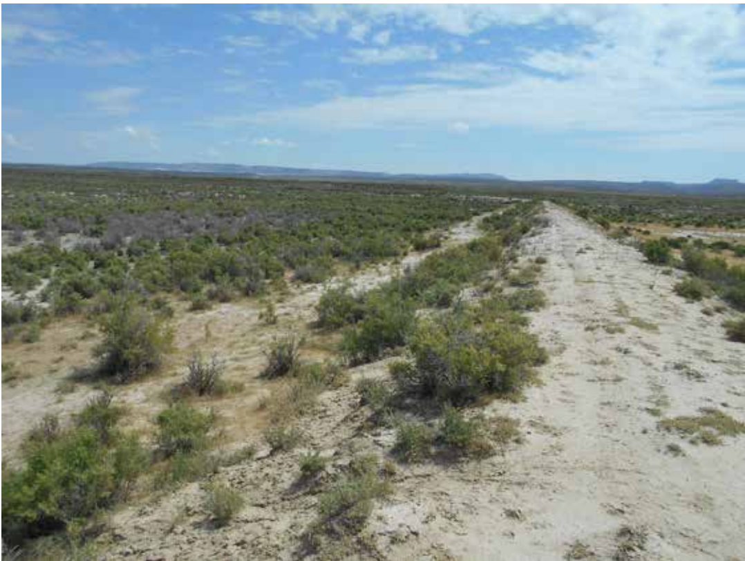
Fifteenmile Reservoir embankment and breach
