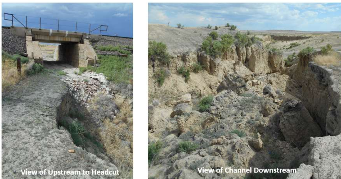
Figure 4.2-34 Headcut at Union Pacific Railroad Crossing.
