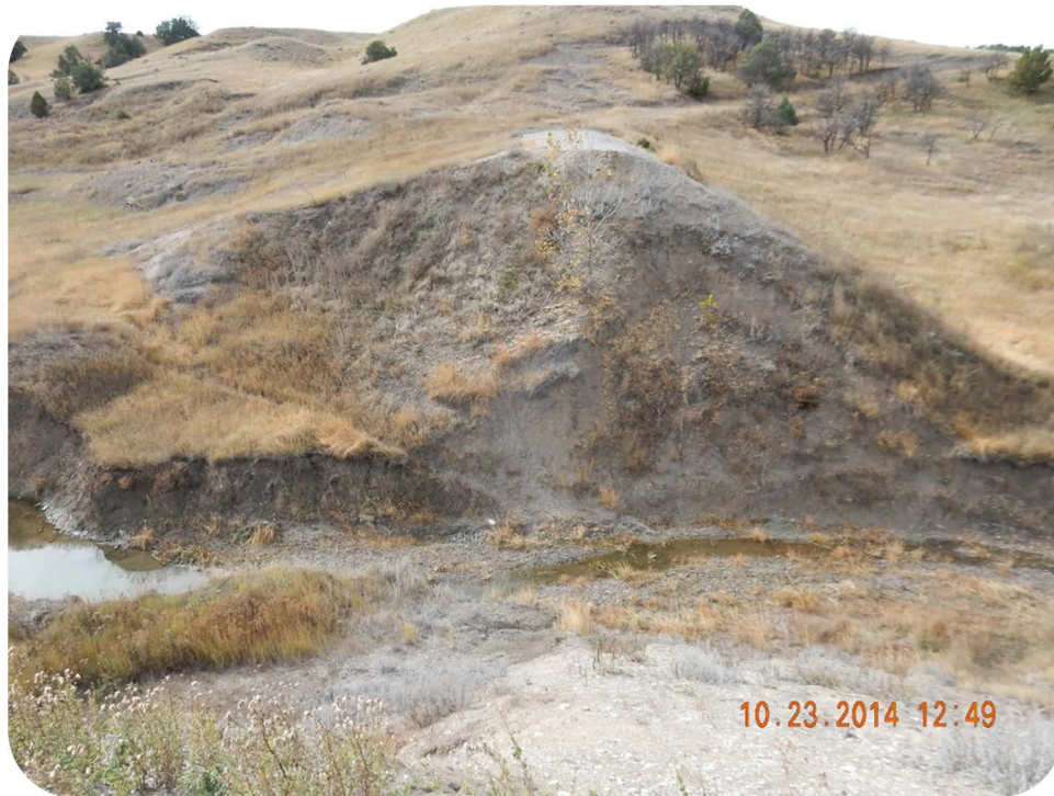
Figure 4.9. A View of Pine (Deep) Creek Reservoir's Breached Dam.
