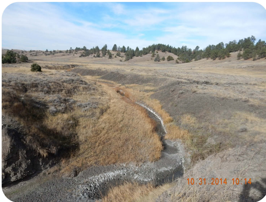
Figure 4.18. A View Upstream of the Breached Dam at the Christofferson Draw Storage Site.
