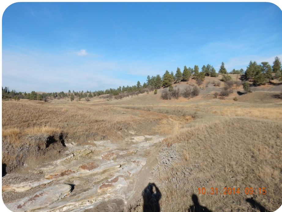
Figure 4.20. A View Looking Upstream From the Breached Dam at the Mule Shoe Storage Site.
