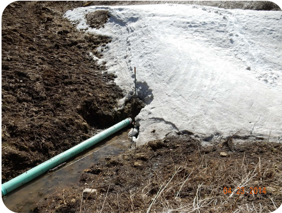
Figure 4.3. Diversion Outlet Pipe on Sunset Reservoir (Hemler Dam).
