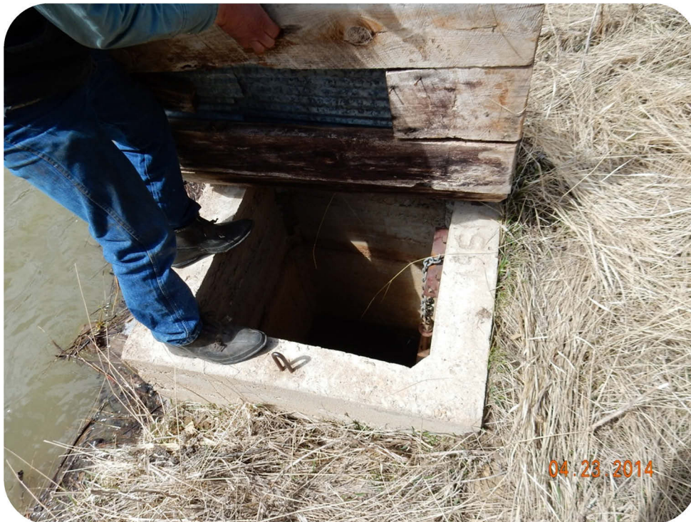
Figure 4.4. Diversion Control Diversion Structure on Sunset Reservoir (Hemler Dam).
