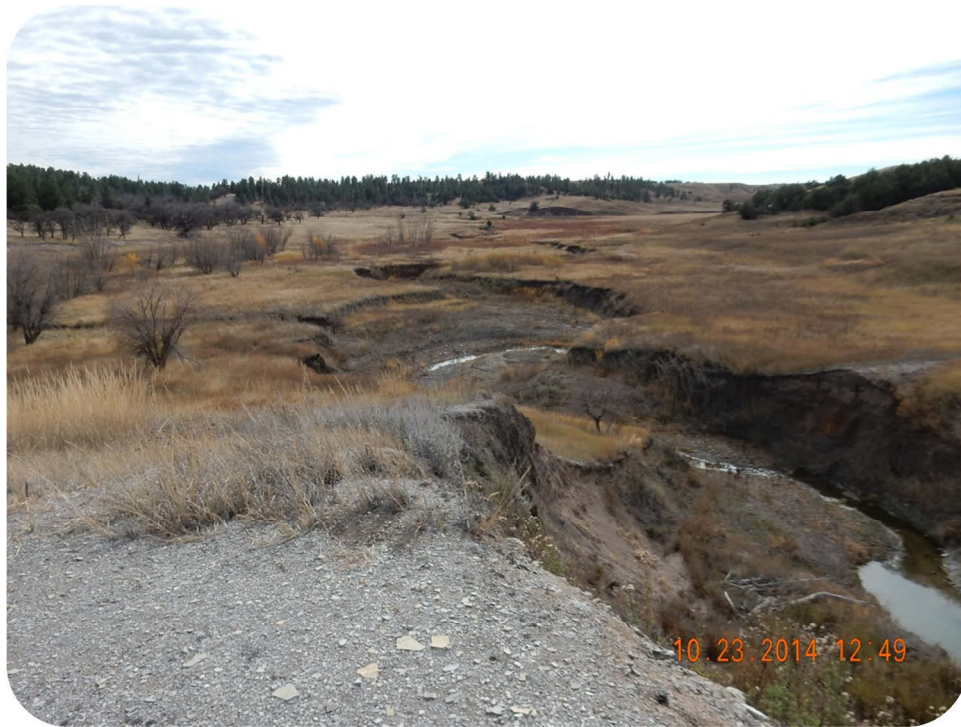
Figure 4-85. A View Looking Upstream From Pine (Deep) Creek Reservoir's Breached Dam.
