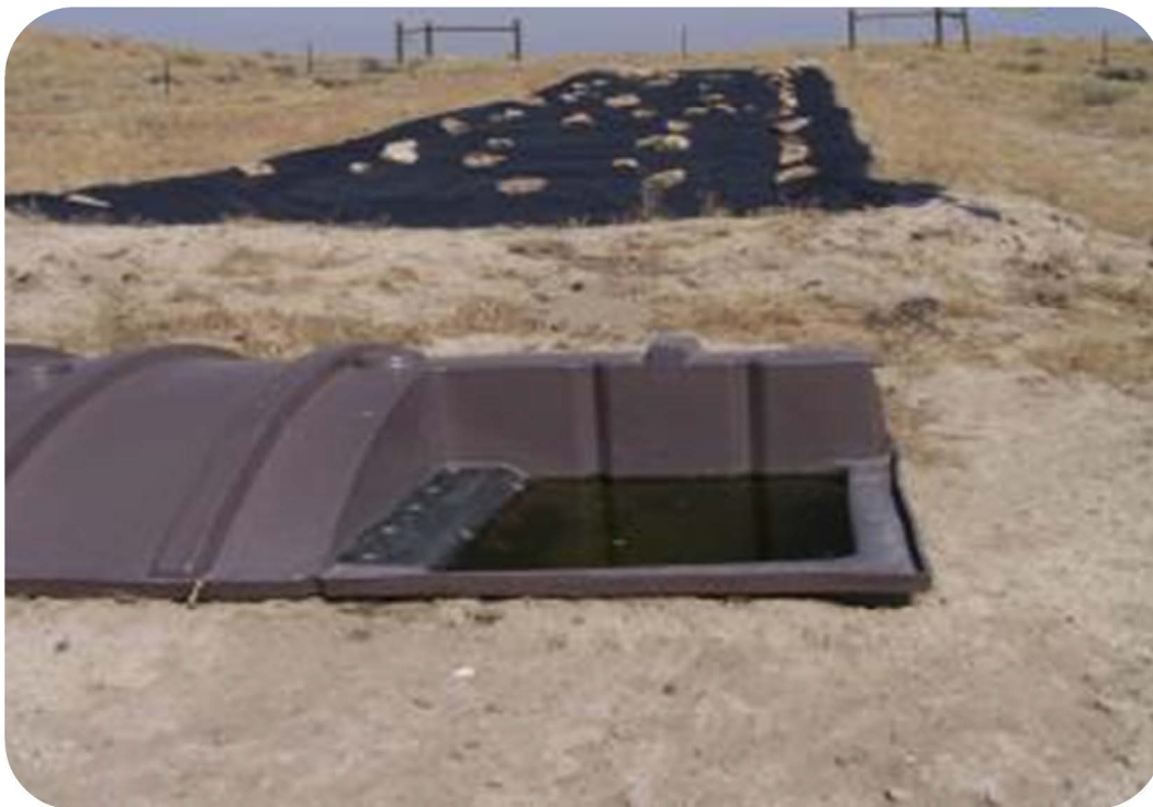
Figure 4-70. An Example of an Installed Wildlife Guzzler System.
