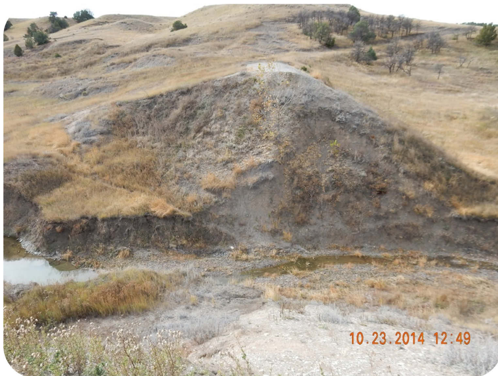
Figure 4-86. A View of Pine (Deep) Creek Reservoir's Breached Dam.
