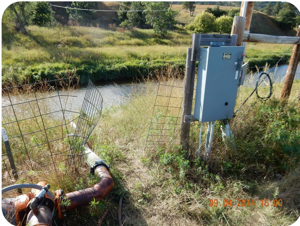
Figure 4-4. Irrigation Pump and Diversion Structure on the Belle Fourche River.
