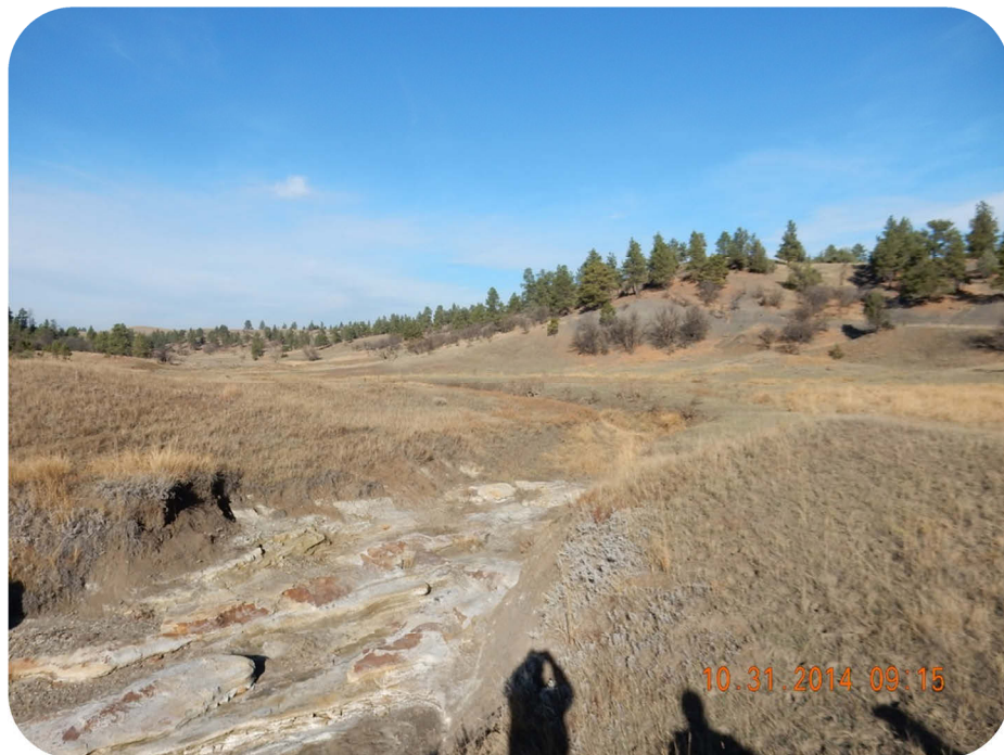
Figure 4-97. A View Looking Upstream From the Breached Dam at the Mule Shoe Storage Site.
