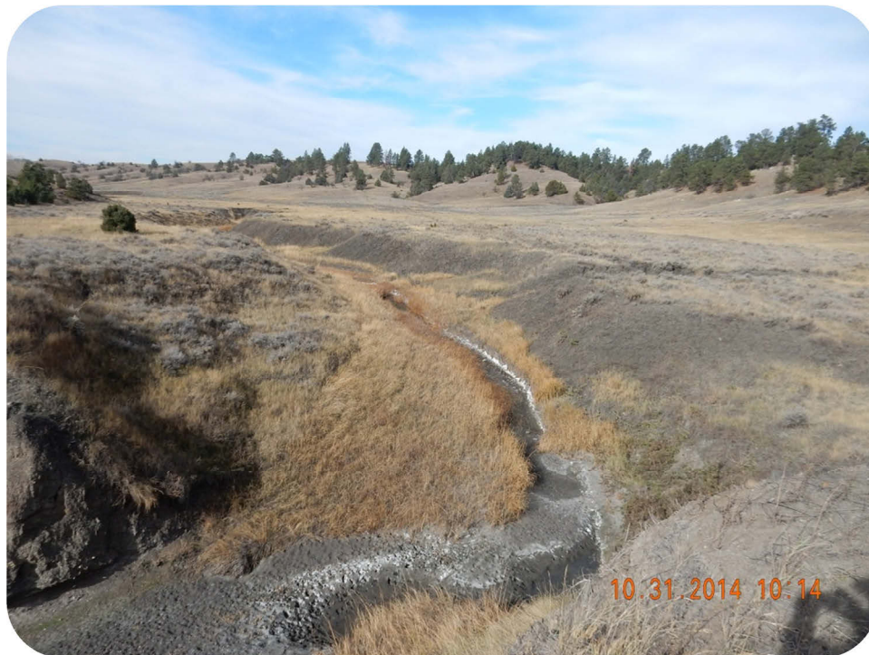
Figure 4-95. A View Upstream of the Breached Dam at the Christofferson Draw Storage Site.
