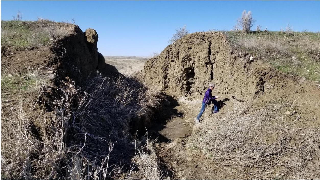
Photo 33 Breached dam proposed for repair (WSS-32.1).
