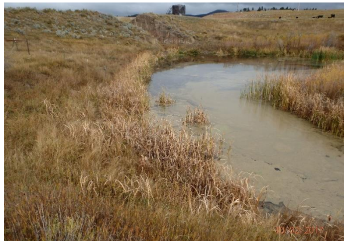
Photo 31 Breached dam for rehabilitation (WSS-8.1).
