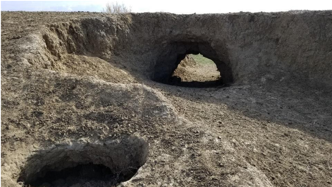
Photo 35 Breached dam (WSS-39.2)
