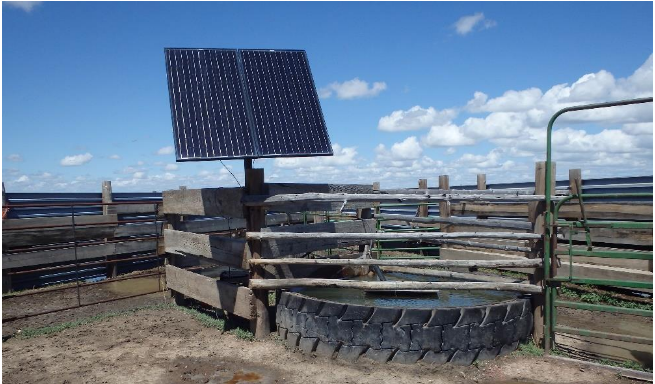
Photo 29 Existing solar well to supply an expanded pipeline and stock tanks (LWW-36.1).
