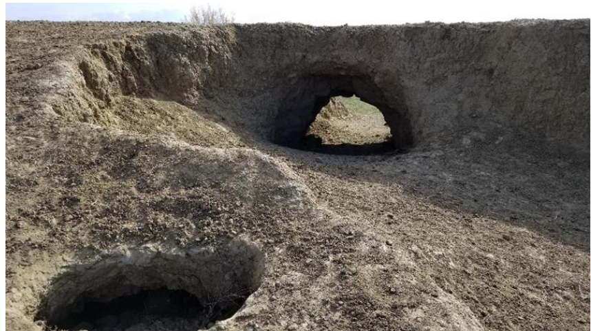
An example of a breached dam recommended for repair.
