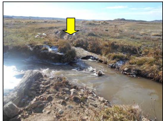
Figure 3.3-6 Inoperable Irrigation Headgate on Bridger Creek.
