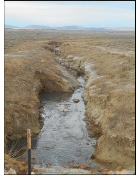
Figure 3.6-12 Channel degradation associated with discharge of oil and gas process water.
