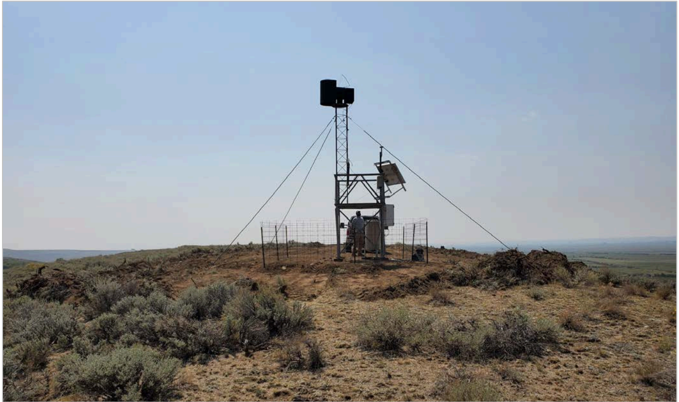
Figure 19. Installation of Willow Lake (equipment relocated from Sweetwater) was completed on 30 August 2021. Thank you to the landowner for grading the road and preparing the surface area, it was greatly appreciated! Photo by WMI Technician Michael Paul.
