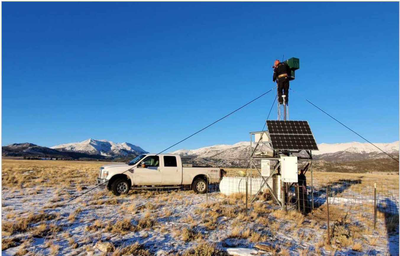
Figure 11. The WMI technician crew preform a maintenance check of generator WR03 (White Acorn Ranch) on 02 December 2020. Replacing the burner nozzle is Patrick Trujillo. Photo by WMI technician Michael Paul.
